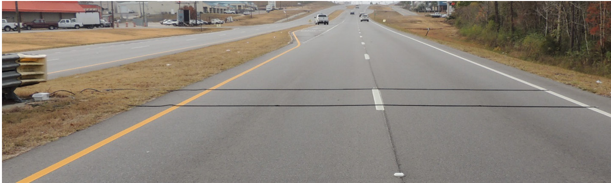
Figure A1. Example of road tubes installation.
