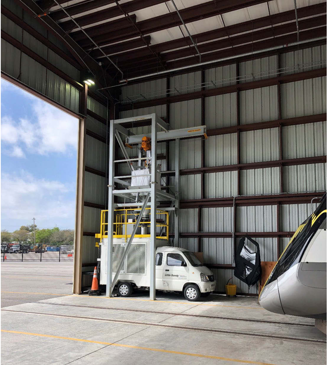
Figure 45: Maintenance building's perimeter enclosure: horizontal steel braces and vertical studs and attached corrugated metal sheets
