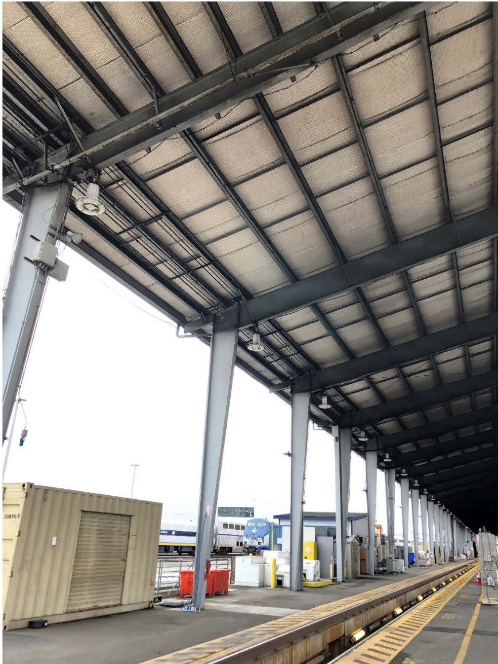
Figure 12: Structural components of the outdoor light facility: Steel portal frame and roof system and maintenance pit
