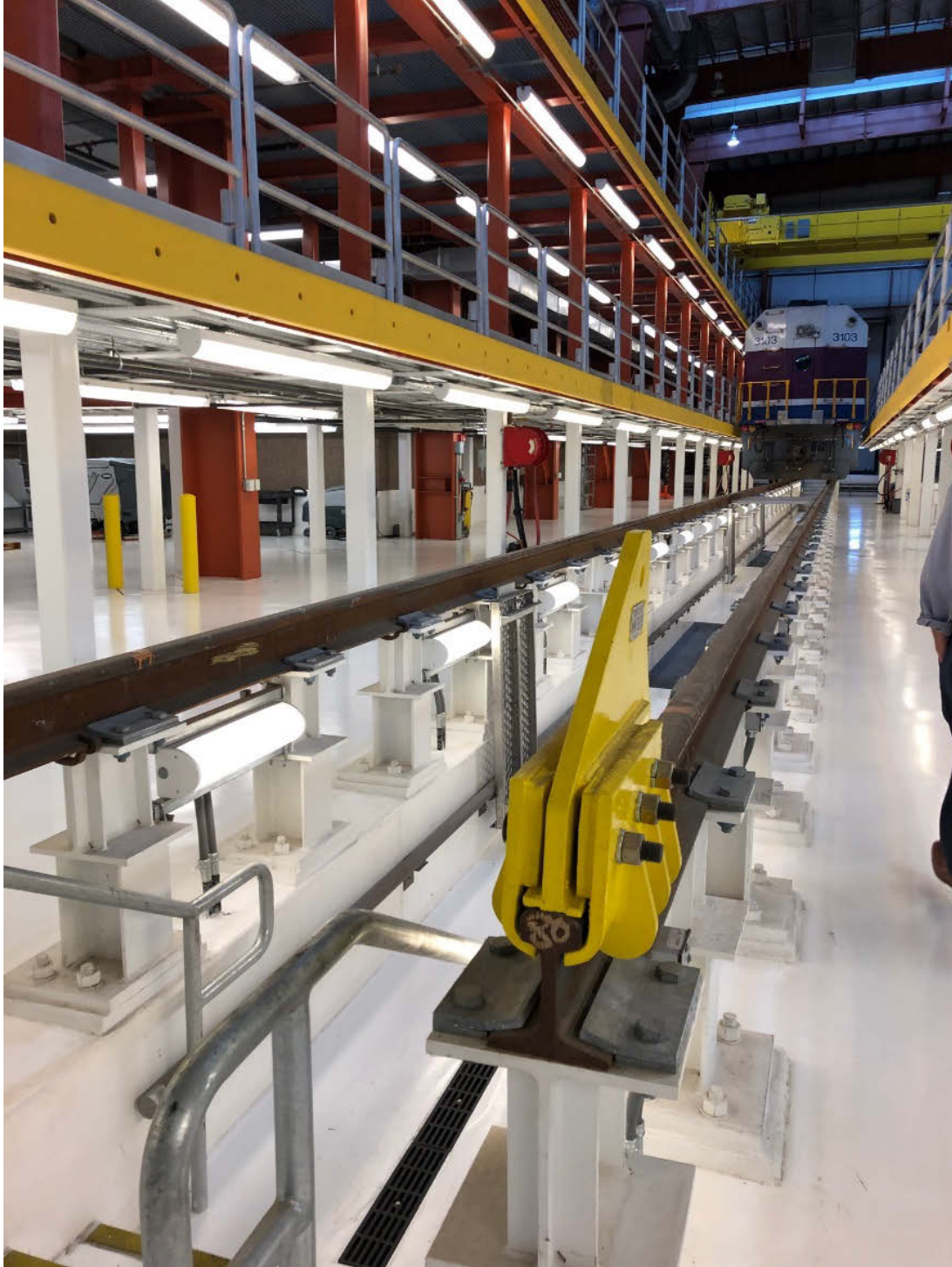
Figure 19: Raised steel deck flooring seated on steel HSS columns and the raised track supported on H-shape steel piers
