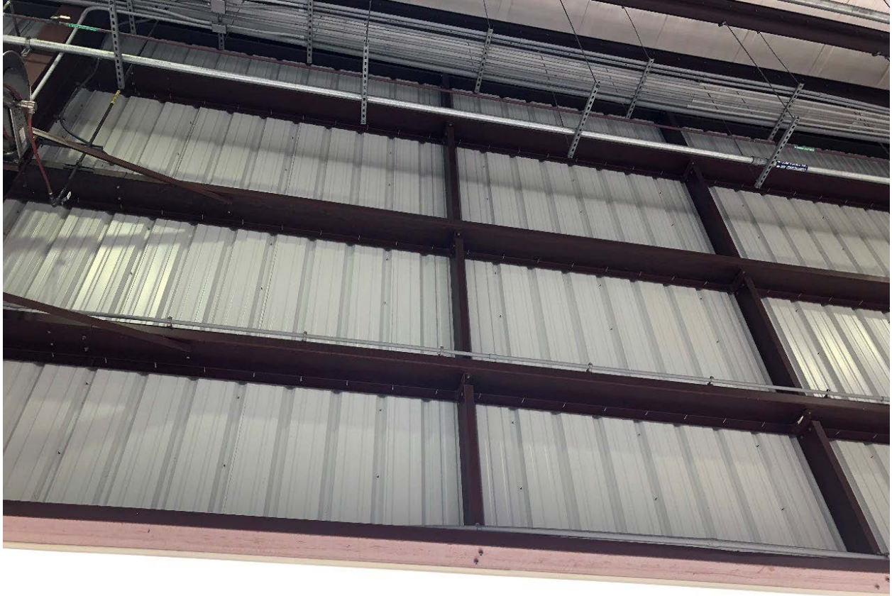
Figure 46: A close view of the facility enclosure: The horizontal steel braces and the attached metal sheets
