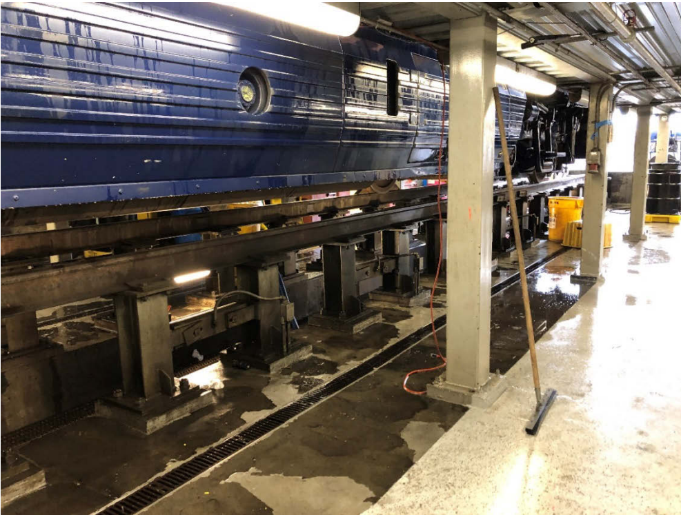
Figure 11: Raised steel deck flooring on steel HSS columns and the raised track supported on H-shape steel piers
