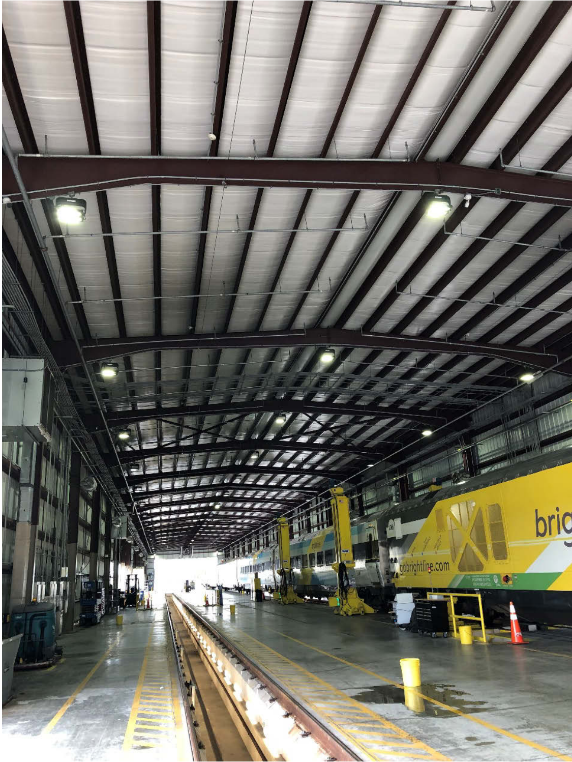
Figure 44: Building structural components: steel portal frame, concrete slab on grade, and the maintenance pit
