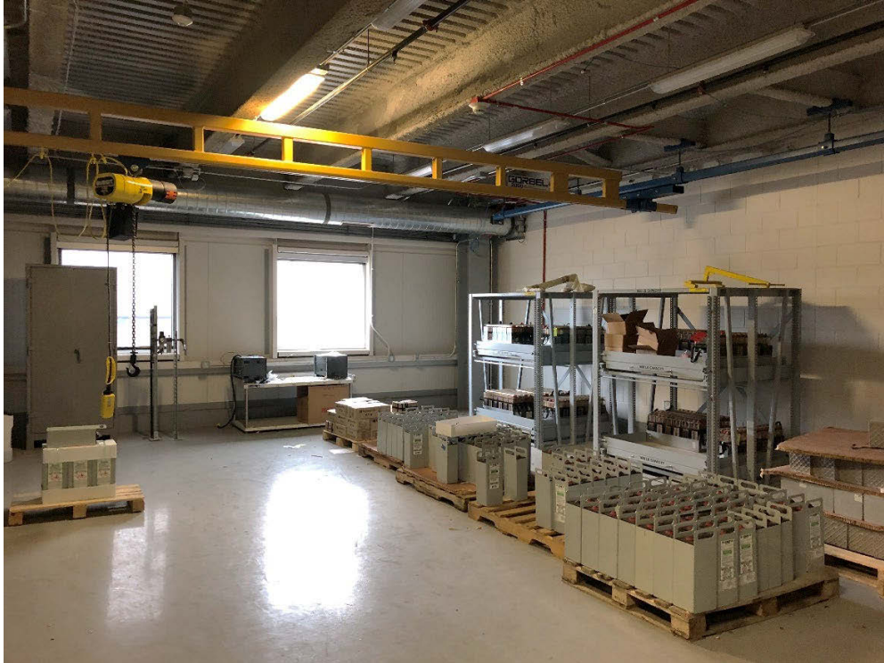
Figure 32: Small capacity overhead cranes installed in the shop rooms
