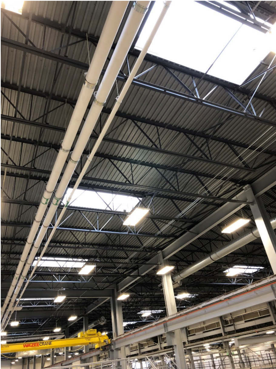
Figure 28: Building's structural components: Steel columns and girders and roof truss-joists spanning east-west
