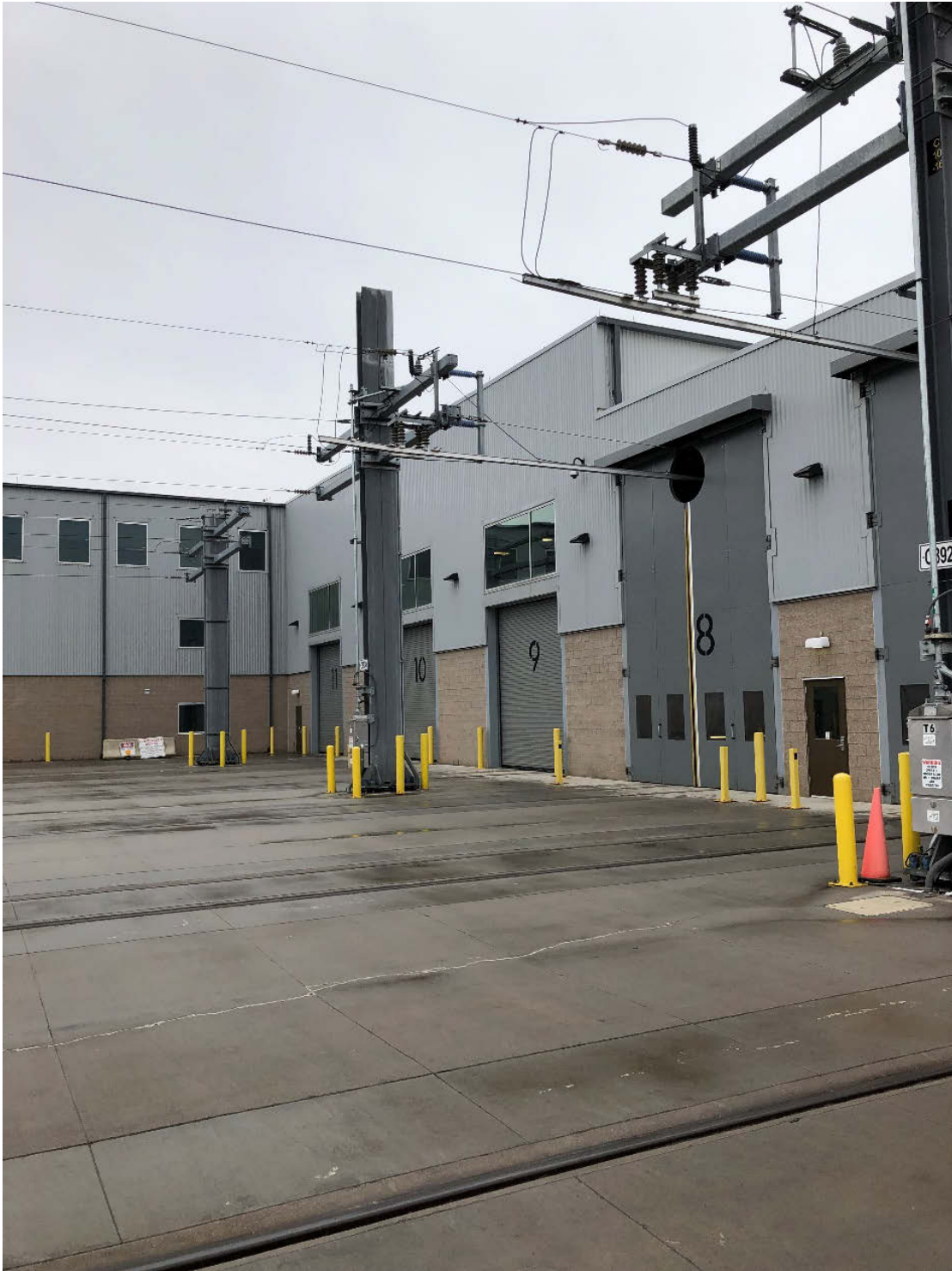
Figure 35: The facility's doors – Roll-up aluminum doors for regular tracks and tall double-fold steel doors for powered tracks
