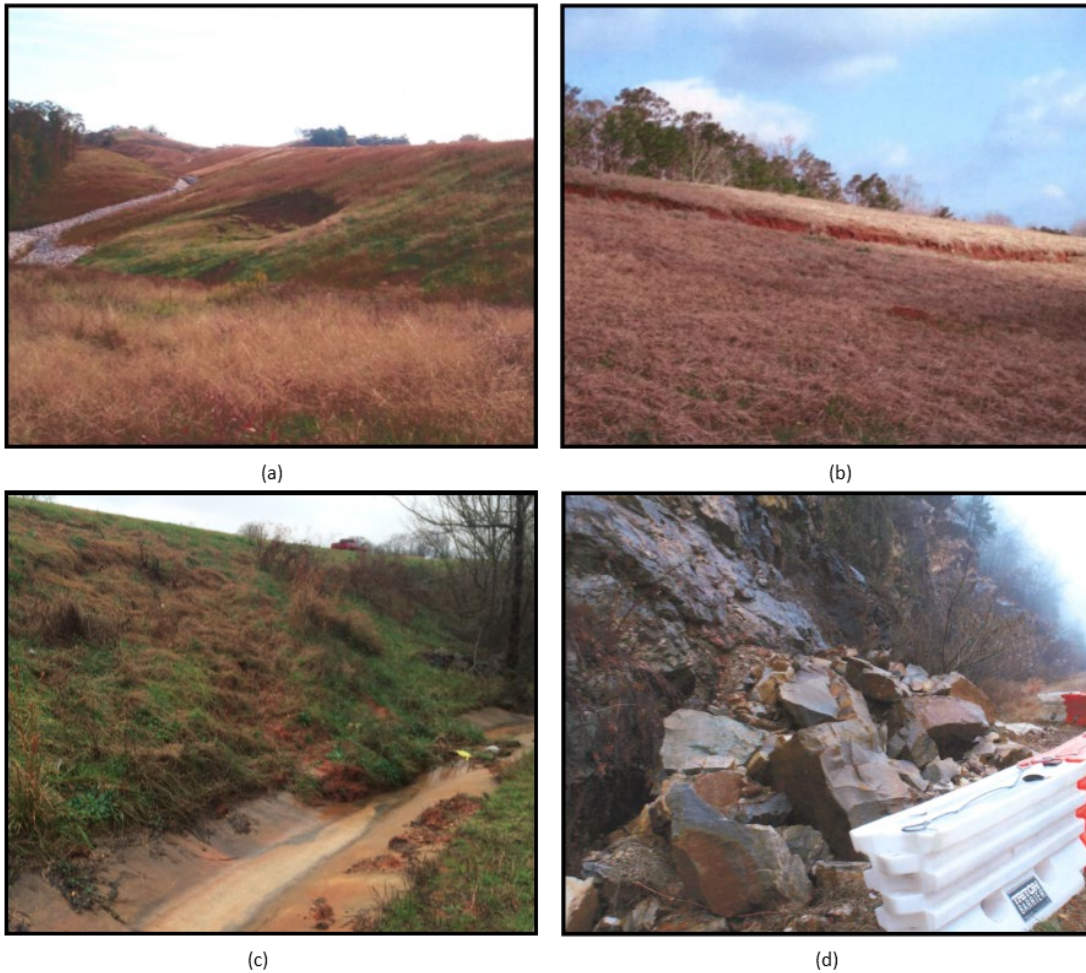
Figure 1-1. Different types of landslide movements observed along Alabama highways including: (a) an earth rotational landslide (b) an earth translational landslide, (c) a surface erosion (creep) failure (d) a rock fall.
