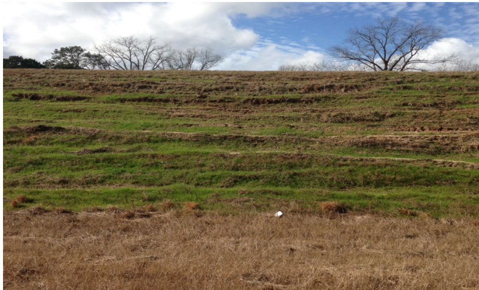
Figure 3-5. Rutting along the face of a slope due to mowing activities (photo provided by Jacob Hodnett, ALDOT).
