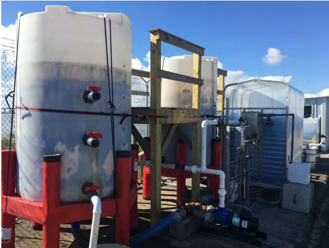
Figure 3-3 Decant and Feed Tanks and Transfer Pump
