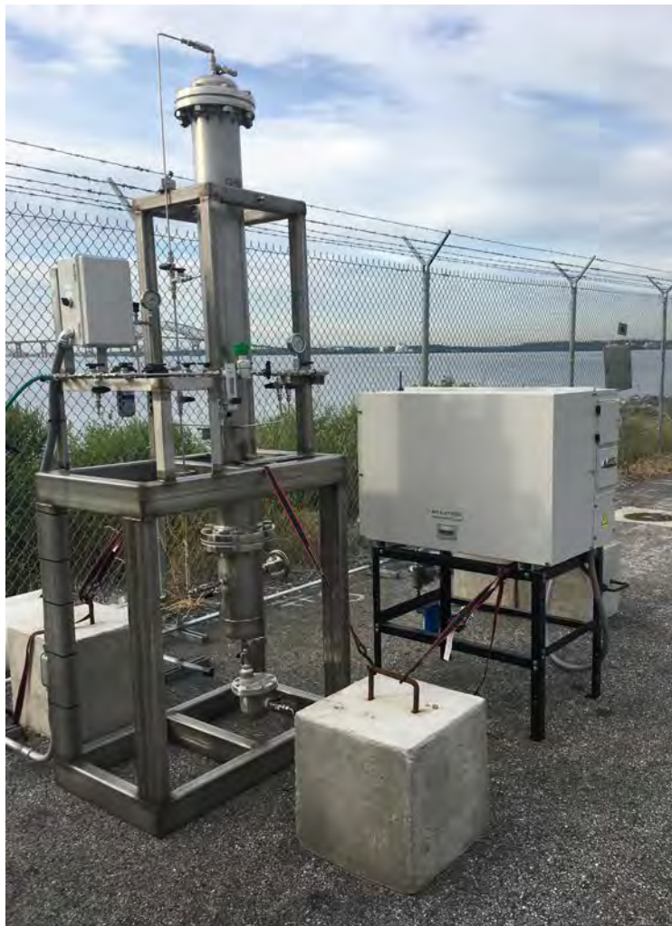
Figure 3-13 Fuel Cell on Site Adjacent to Gas Conditioning and Compression Unit
