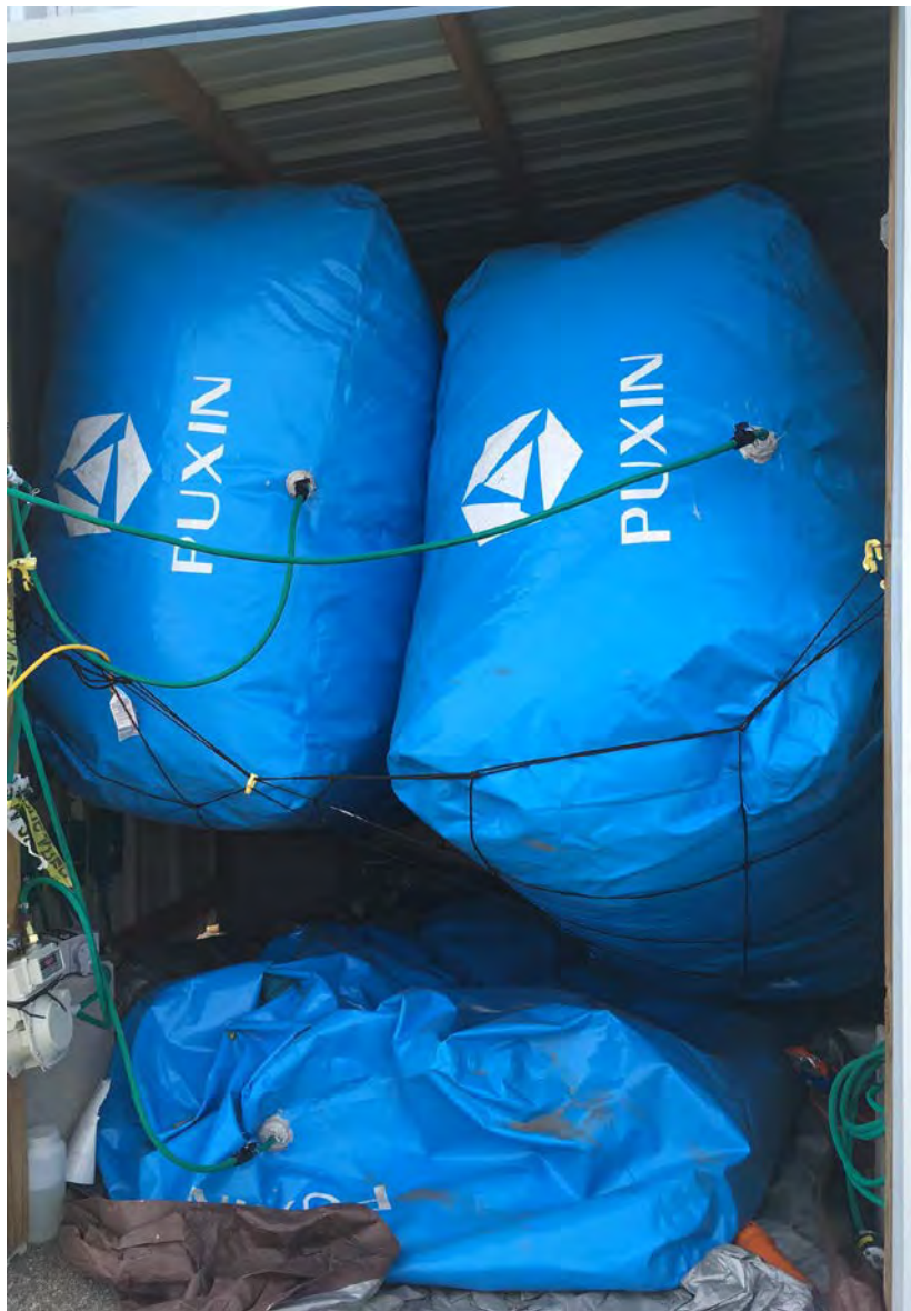
Figure 3-7 External Biogas Storage Bags
