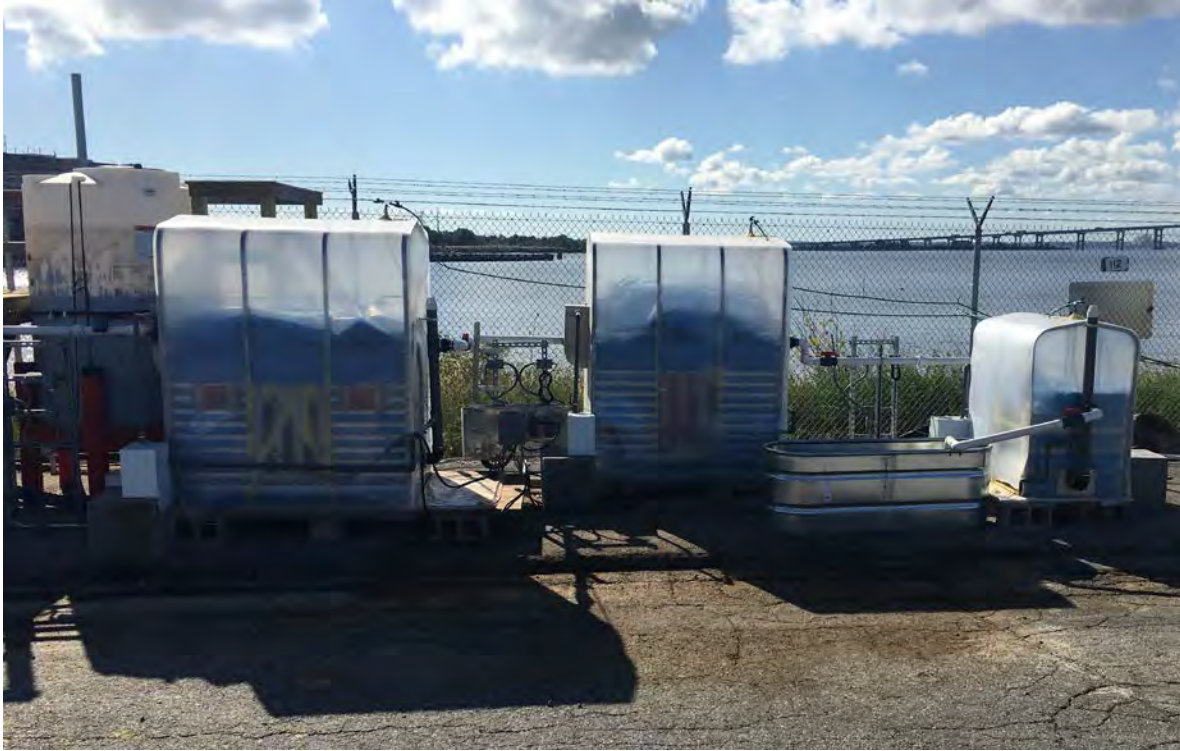
Figure 3-6 Three Algal Digesters and Open Digester Effluent Receiving Tank
