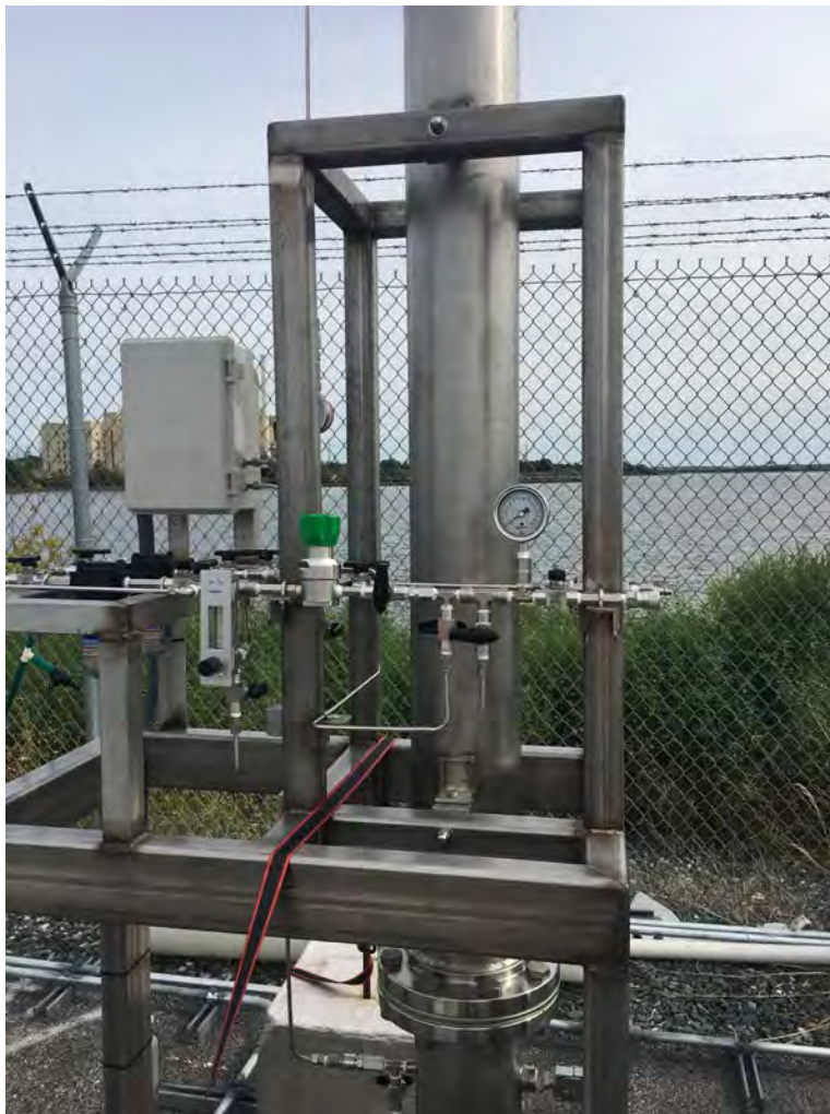
Figure 3-10 Front View of Biogas Conditioning and Compression Unit
