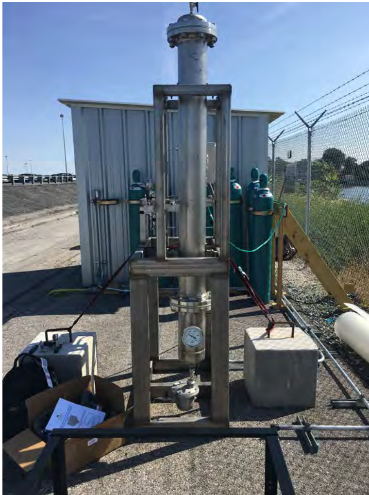
Figure 3-9 Side View of Biogas Conditioning and Compression Unit
