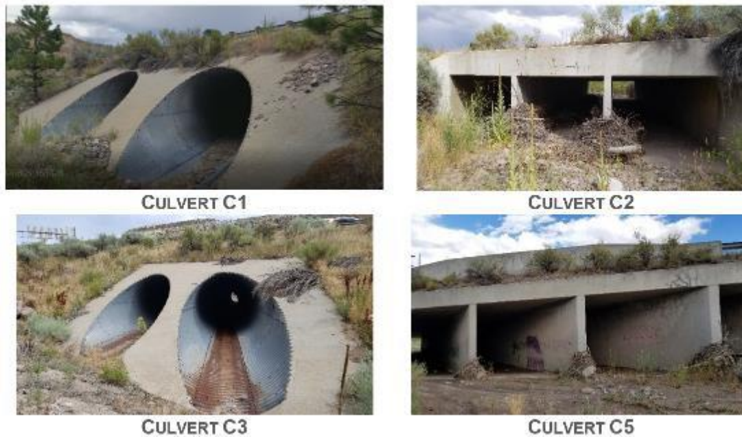
Figure 4. Three culverts were selected for analysis based on data availability (C1, C2, and C3).
