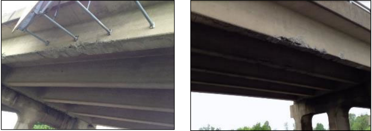
Fig. 19. Damage to concrete girders
