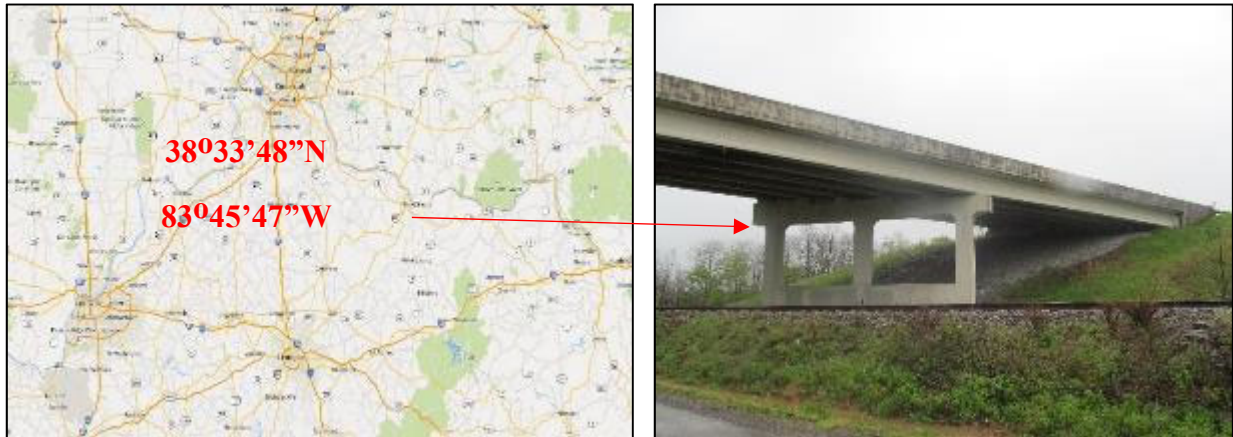
Fig. 24. Location of KY 11 over CSX railroad and Strodes Run Pike in Mason County, KY
