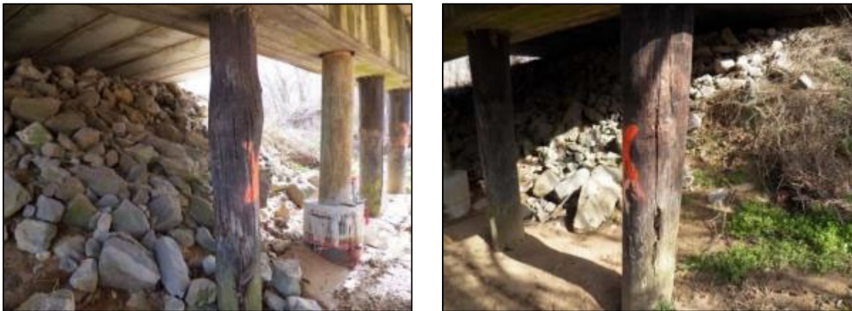
Fig. 40. Typical damage to KY 339 timber pile supports
