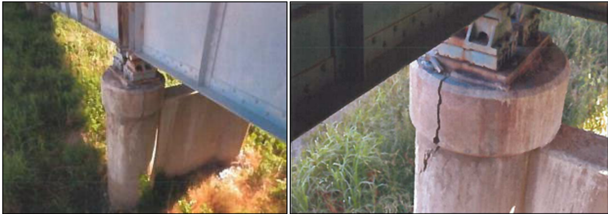
Fig. 34. Typical damage to pier cap in US 60 bridge over Cumberland River
