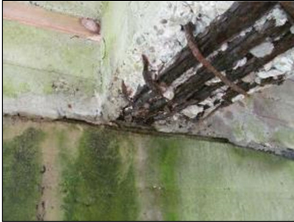
(a) Damage observed in girder G2
