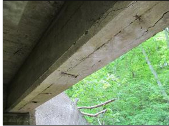
(b) Longitudinal cracks in girder G1
