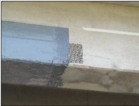
(a) Finger joint of CRP 070 left void of epoxy
