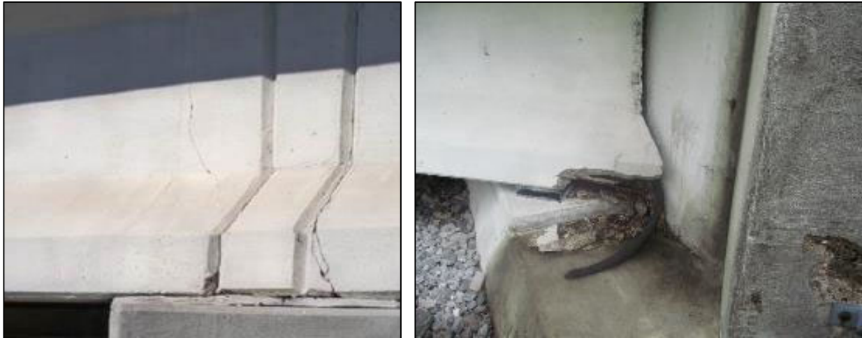
(a) Cracks at PC girder ends
