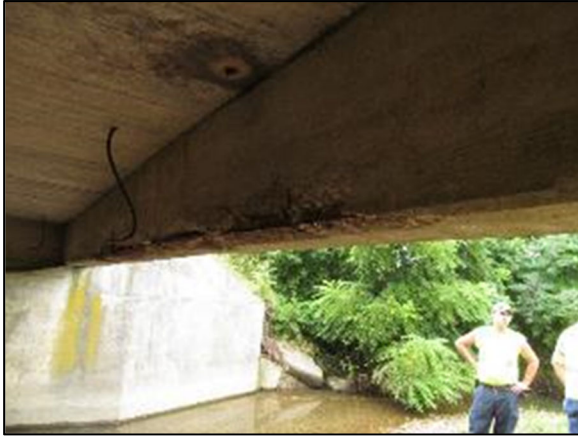
(a) Damage to girder G1
