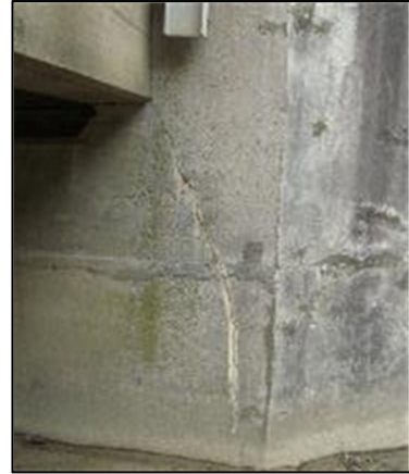
(b) Damage to abutment wall
