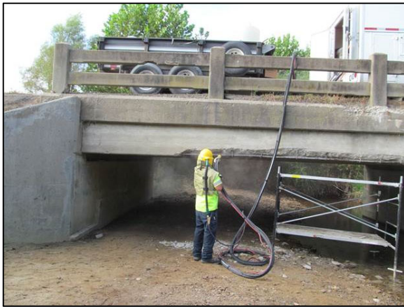
(c) Sandblast exposed steel rebar
