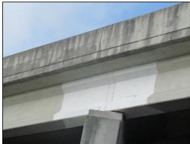
Fig. 31. Completed repairs on either side of Pier 1 following application of protective coating
