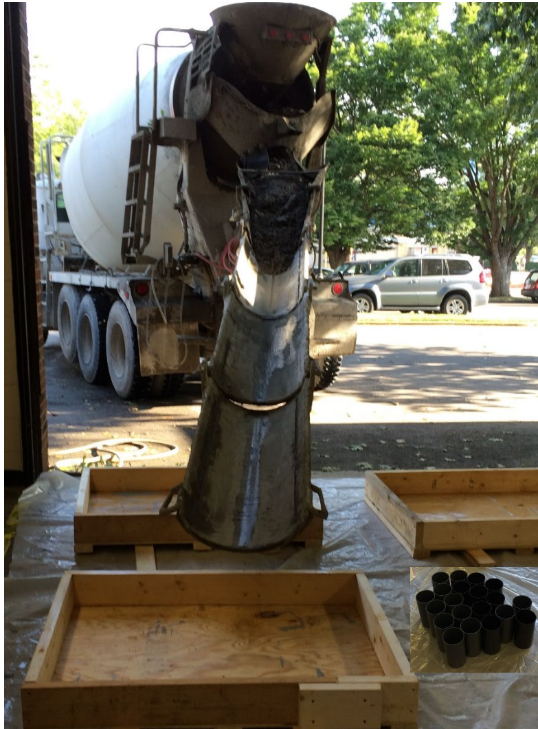
Figure 1 Three (3) concrete slabs with dimensions of 30.5" (width) x 46.5" (length) x 5.5" (depth) and twenty (20) 4" (diameter) x 8" (length) cast-in-place cylinder modal concrete samples are poured in the garage.
