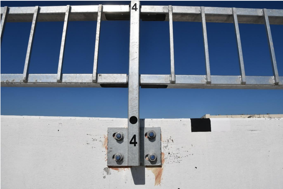
Figure 6. 2020 MnDOT Bicycle and Pedestrian Rail Spindle with Back of Tube Positioning, Test No. MNPD-3
