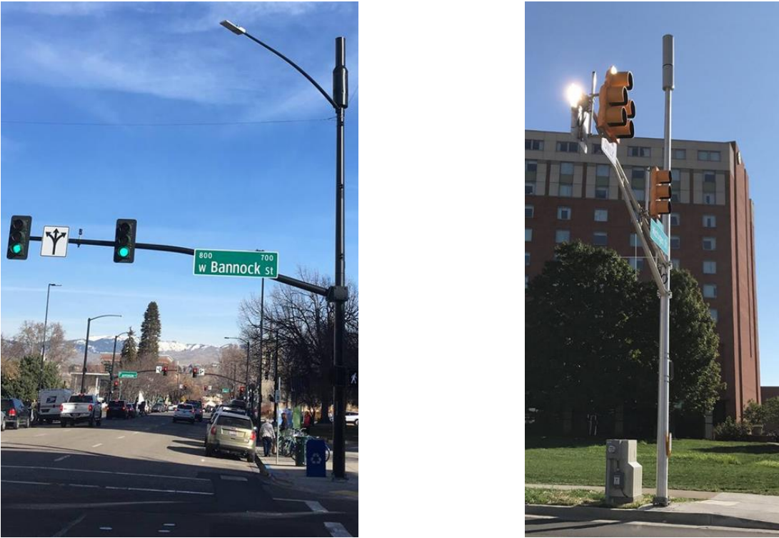
Figure 13. Small cells installed on traffic signals (Left to right: EMI, 2019; NYM, 2020).
