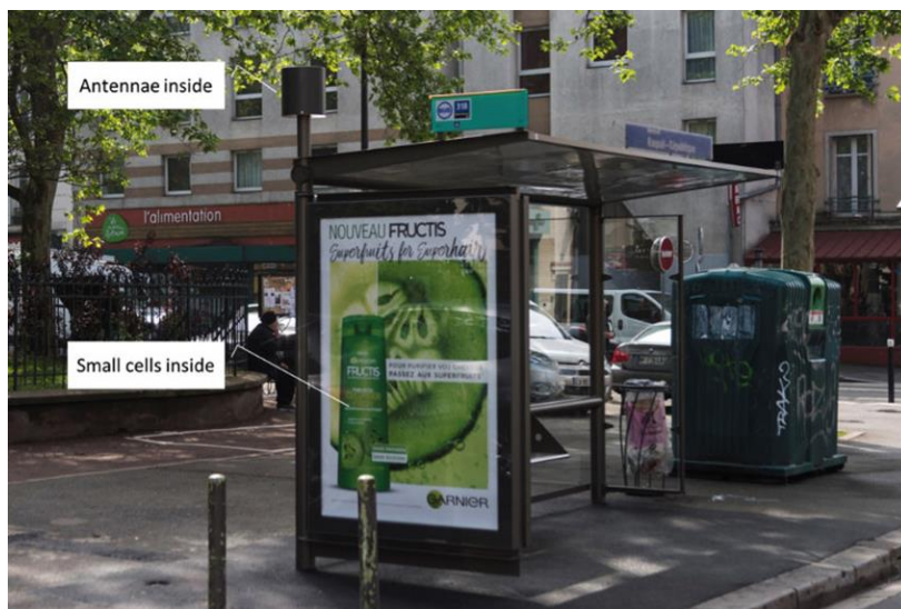
Figure 16. Small cells installed inside an advertising board at a bus shelter (ThinkSmallCell, 2017).
