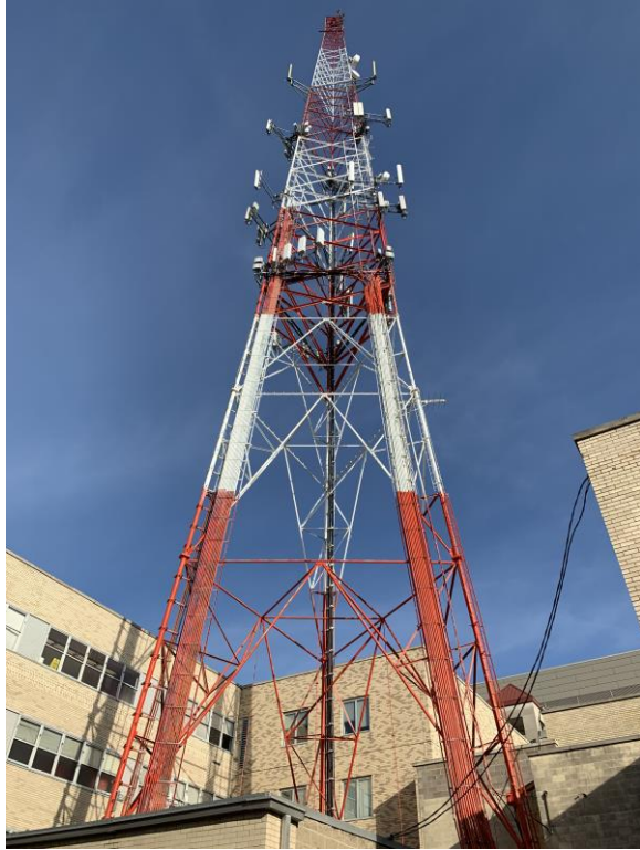
(a) A macrotower holding multiple antennas operated by various cell phone providers.
