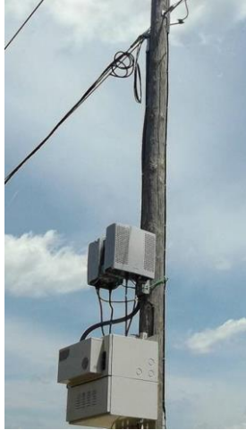
(a) A small cell and utility boxes are installed at the mid-location of a utility pole (Daily Herald, 2018).
