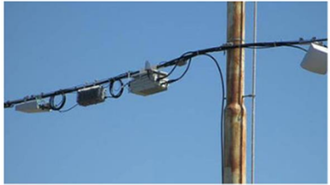
(b) Small cells and utility boxes are hung from power lines (Wade4Wireless, 2015).
