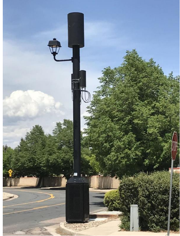
(b) A small cell attached at the top of a streetlight pole (Heilman, 2018).
