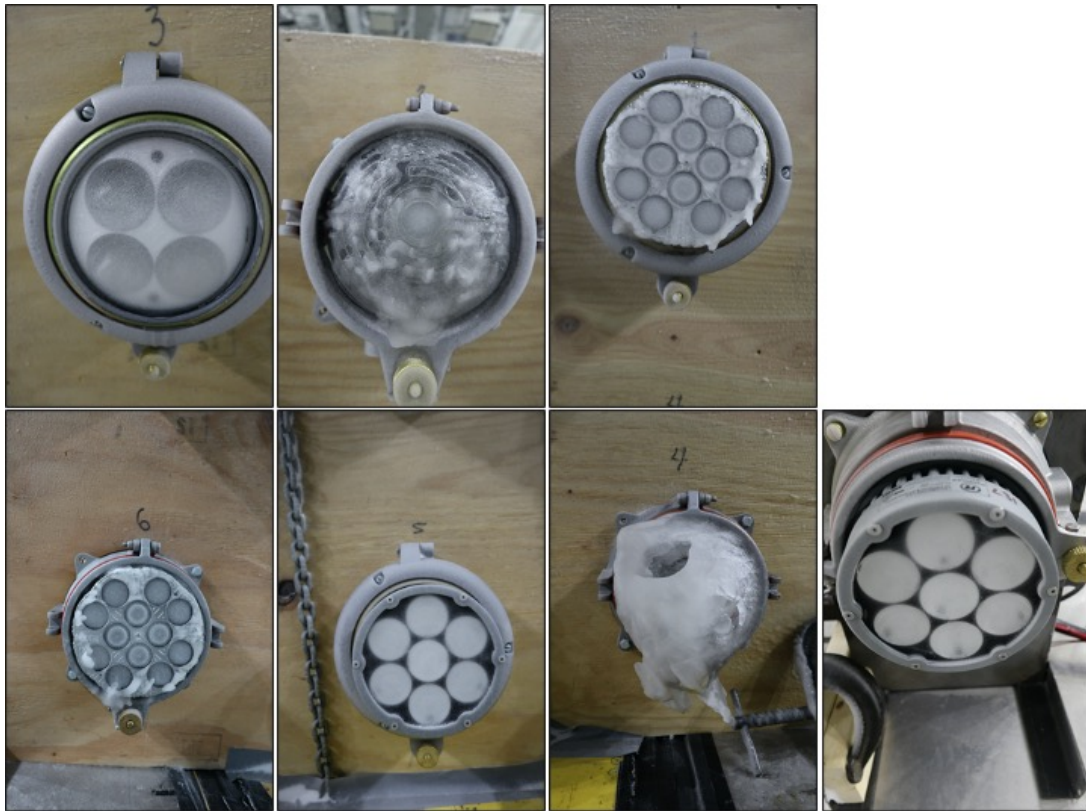
Figure 15. Close-up view of the accumulation of snow and ice on light fixtures after Trial 1
