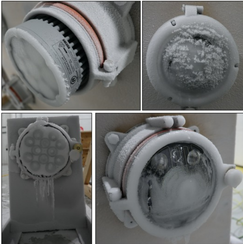
Figure 10. LED light fixtures after 30 minutes of operation at -20 °C
