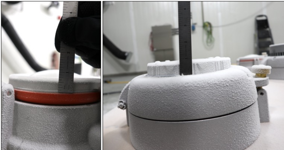
Figure 5. Light fixtures with 1/4-inch accumulation of ice
