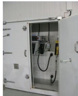
In-chamber refueling station
