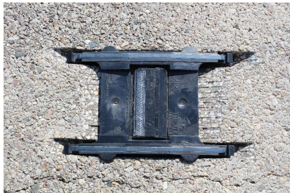
Figure 9. Marker placed in dry cut (no adhesive) to verify leveling tabs rest on the pavement.
