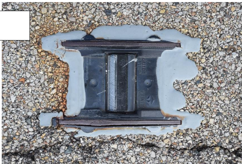
Figure 23. Example of Guide Lite with leading edge of rail exposed after one year.
