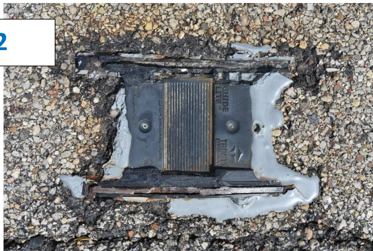
Figure 27. Guide Lite marker in very poor condition after two years of service on I-155.
