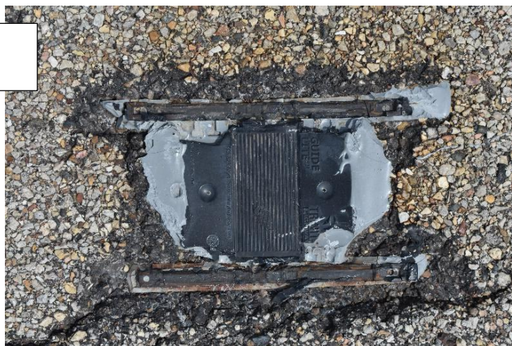
Figure 20. Guide Lite with no lens after two years of service on I-155 (central HMA site).
