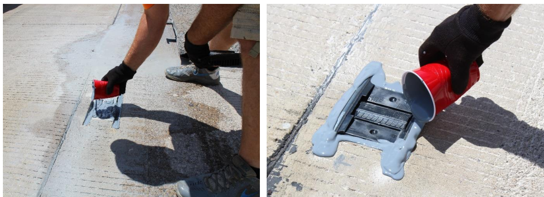
Figure 10. Epoxy adhesive being poured before and after the marker is placed in the cut.
