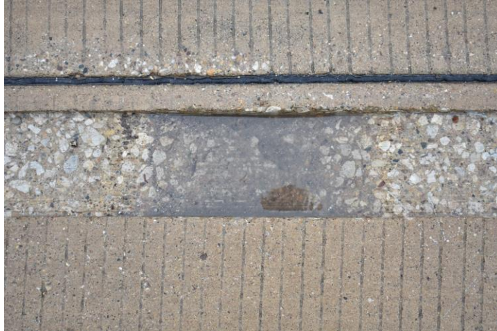
Figure 17. Missing R-100 on IL-8 (central PCC site).
