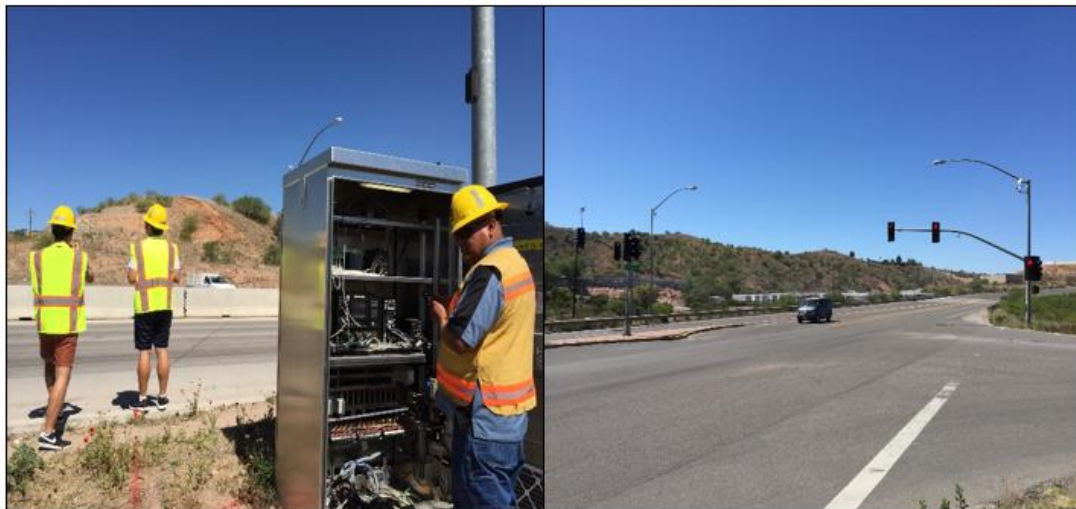
Figure 8. Site Visit to SR 189, and Intersection of SR 189 and Grand Avenue (November 30, 2016)
