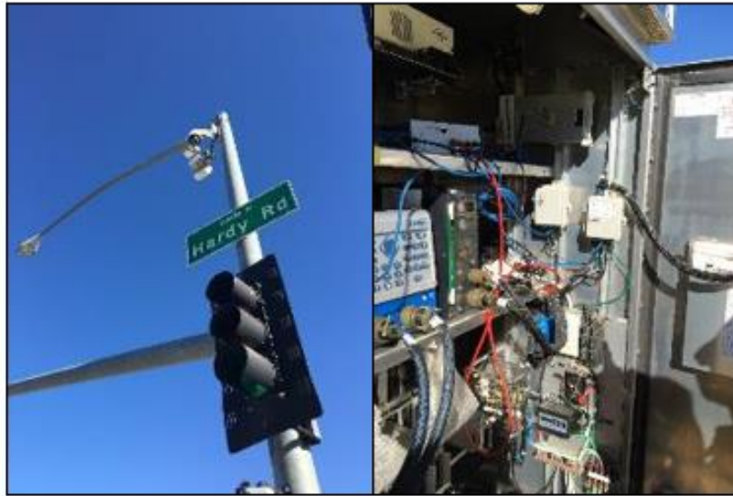
Figure 7. Pole-Mounted Communications and Interior of Traffic Cabinet at Intersection of SR 77 and Hardy Road (September 15, 2016)
