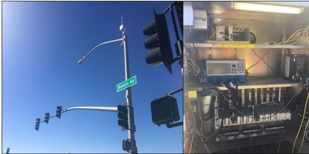
Figure 9. Intersection of SR 347 and Bowlin Road, and Interior of Traffic Cabinet (October 11, 2016)
