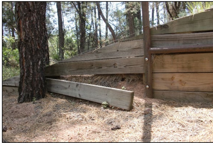
Figure 21. Escape Mechanism in Need of Maintenance
