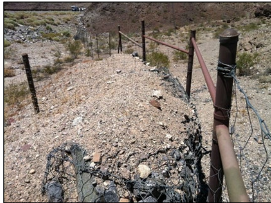
Figure 46. Erosion, Lack of Soil Retention, and Short/Buried Guide Fence
