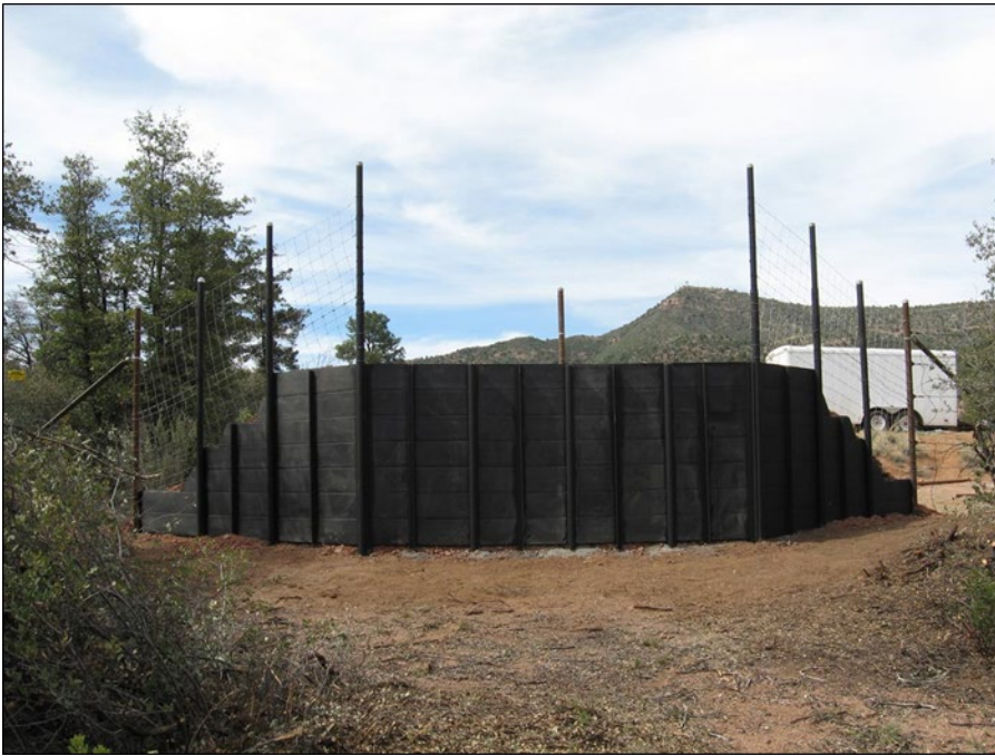
Figure 56. Escape Ramp Using Composite Material to Retain Soil Along State Route 260 in Arizona
