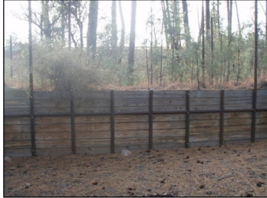
Figure 45. Retaining Wall Too Short to Keep Elk from Entering the ROW (Height Less Than 48 Inches)
