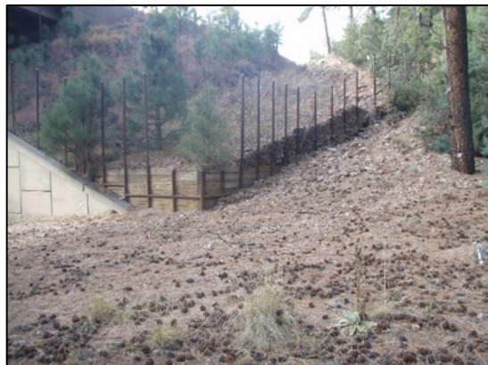
Figure 44. Ramp Placed Near Drainage, Allowing Buildup of Water-Deposited Sediment
