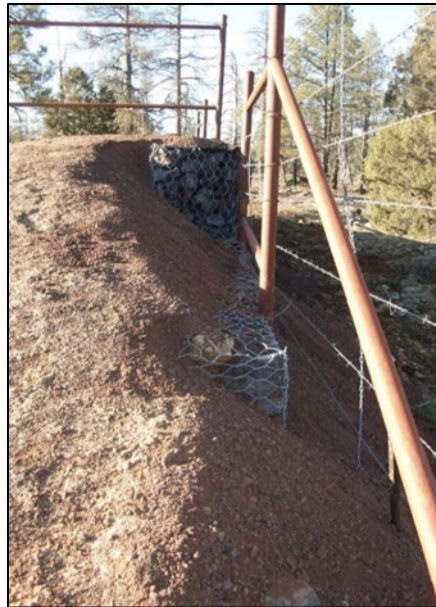
Figure 41. Escape Ramp with a Noncompatible Substrate and No Soil Retention Method
