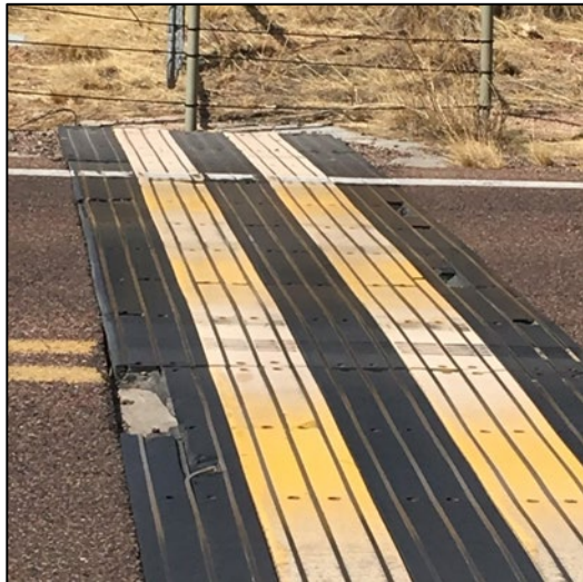
Figure 51. Electrified Mat Material Damaged by Traffic Over Time
