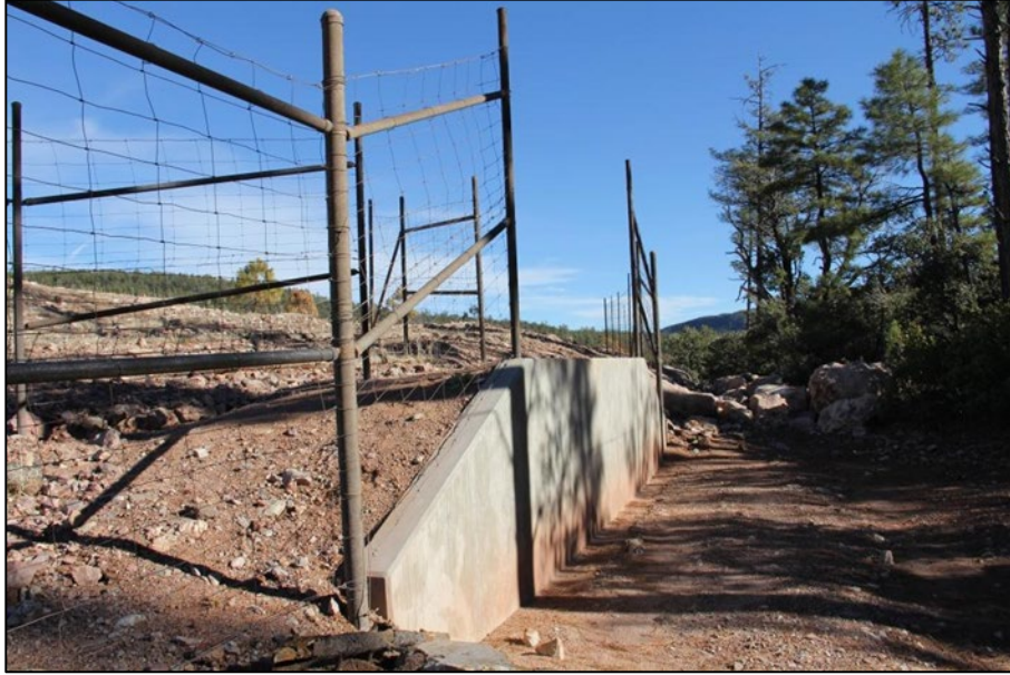
Figure 53. Escape Ramp Using Concrete to Retain Soil Along State Route 260 in Arizona
