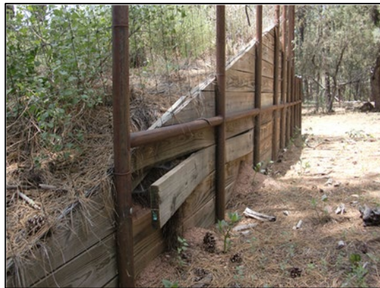
Figure 43. Soil Loss from Failing Wooden Plank Retaining Wall
