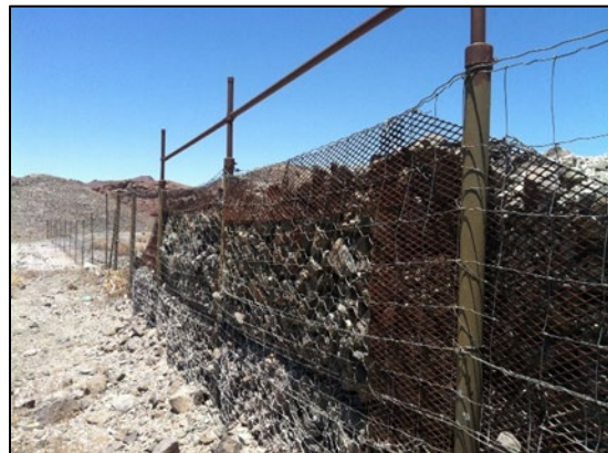
Figure 47. Retaining Mesh Above Lip of Ramp, Creating Potential Escape Obstacle
