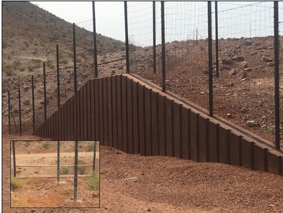
Figure 52. Escape Ramp with Horizontal Bar to Limit Bighorn Sheep Access from Outside the ROW; Inset Photograph Shows Horizontal Bar Detail
