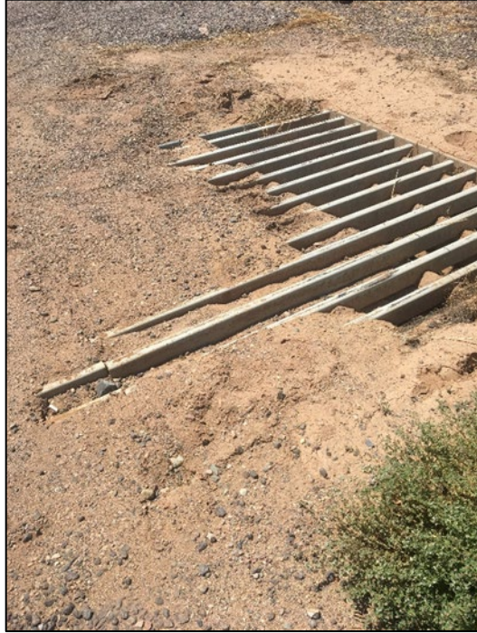
Figure 50. Cattle Guard Partially Filled in with Dirt
