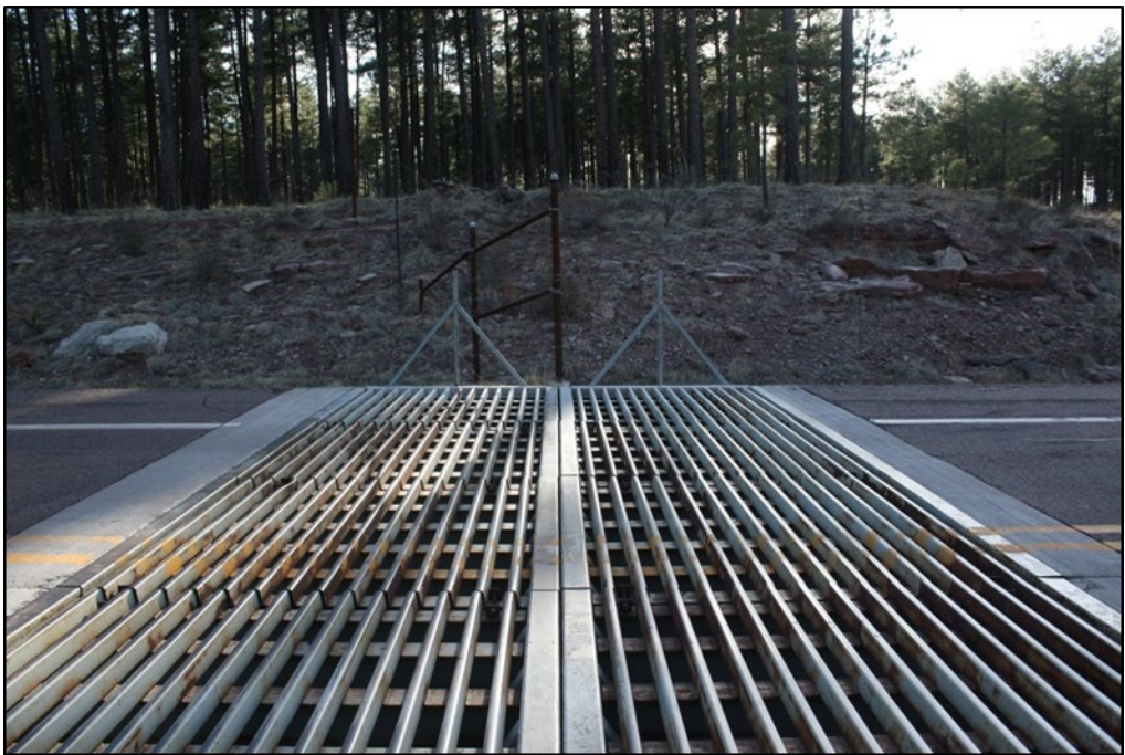
Figure 6. Two ADOT Standard Guards Installed Side-by-Side to Create a Double Cattle Guard
