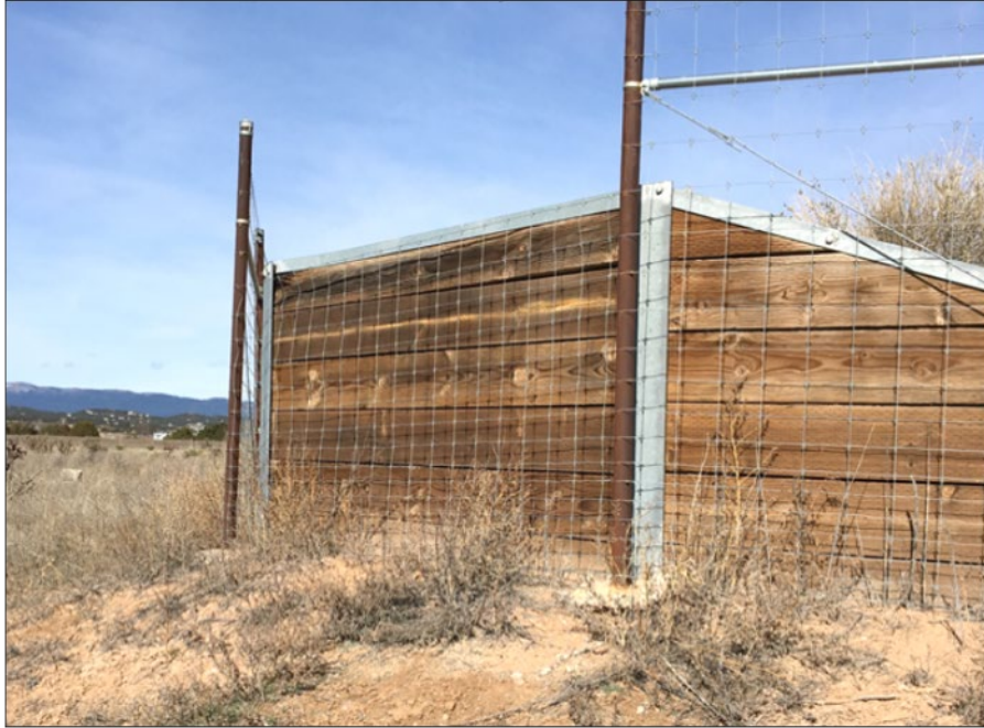
Figure 55. New Mexico Example of Escape Ramp Using Properly Treated and Supported Lumber to Retain Soil Along Interstate 40
