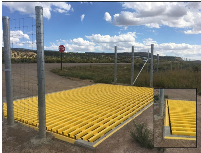
Figure 60. New Mexico Example of Wide Wildlife Guard to Deter Jumping, with Angle Iron Welded to the Vault Edge to Reduce Walking on the Vault Edge, Along U.S. Route 550; Inset Photograph Showing Welded Angle Iron Detail
