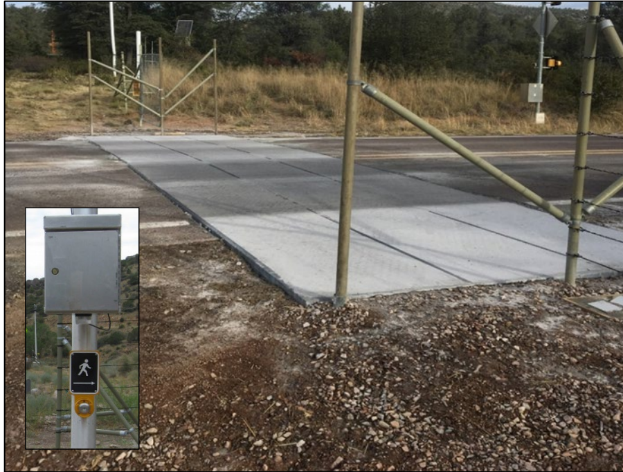
Figure 61. Electrified Concrete Wildlife Guard with Push-Button Power Delay for Pedestrian Crossing Along State Route 260; Inset Photograph Showing Push-Button Detail
