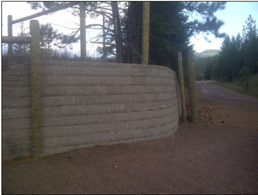
Figure 54. Montana Example of Escape Ramp Using Landscape Blocks to Retain Soil on U.S. Route 93
