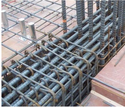
Figure 3. Closely placed shear reinforcement for beam-column joint (courtesy of Gova steel & engineering http://www.govacarports.co.za/index.php?p=2_1_first-page )
