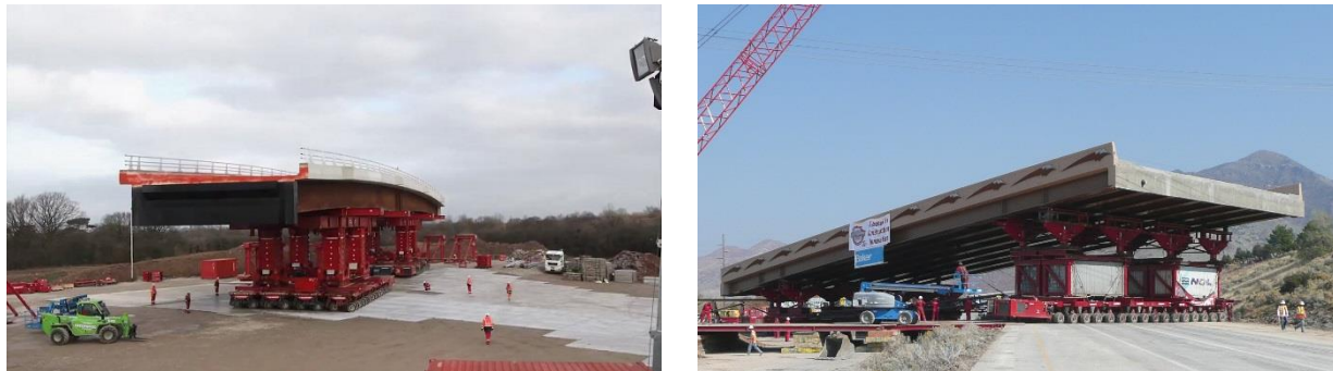
Figure 4. Prefabricated beam elements. Photo courtesy of Utah Department of Transportation ( http://utcdb.fiu.edu/bridgeitem?id=257 ) and Manchester Evening News ( http://www.manchestereveningnews.co.uk/news/greater-manchester-news/incredible-time-lapse-video-shows-new-8920375 )
