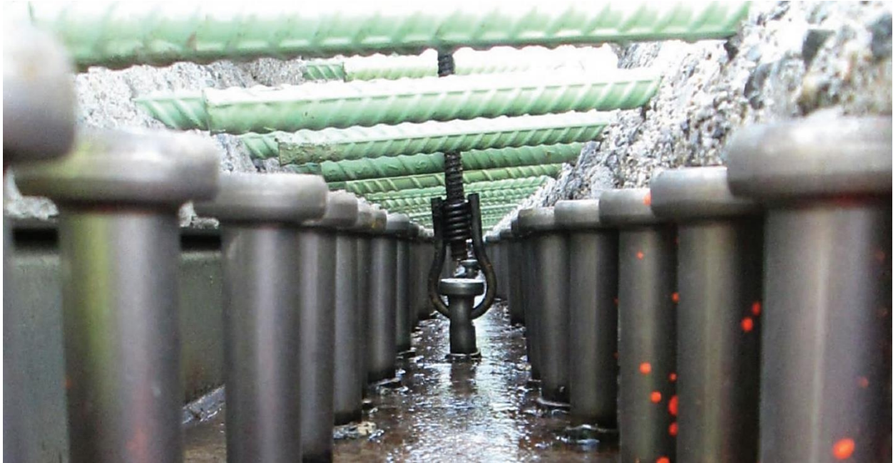
Figure 140. Longitudinal connection detail above first interior girder line with shear studs stopping below the bottom mat of rebar (Ben Graybeal 2014a)
