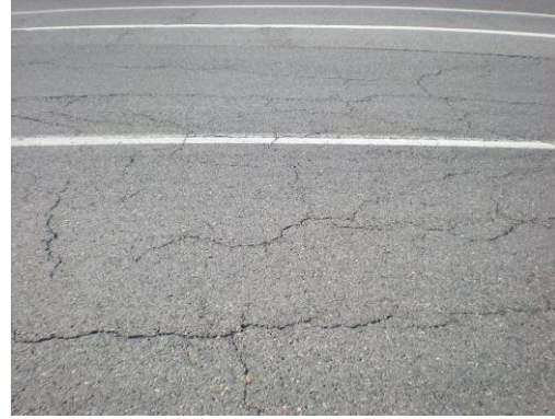
(b) Close up of road showing cracks
