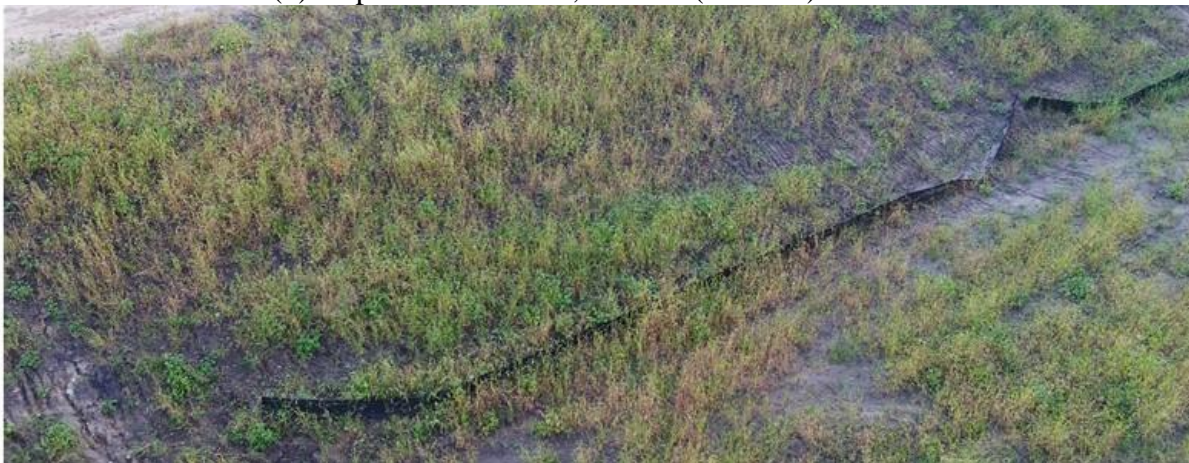
(c) Inspection 9/24/2019, 6.78 in. (17.22 cm) rainfall
