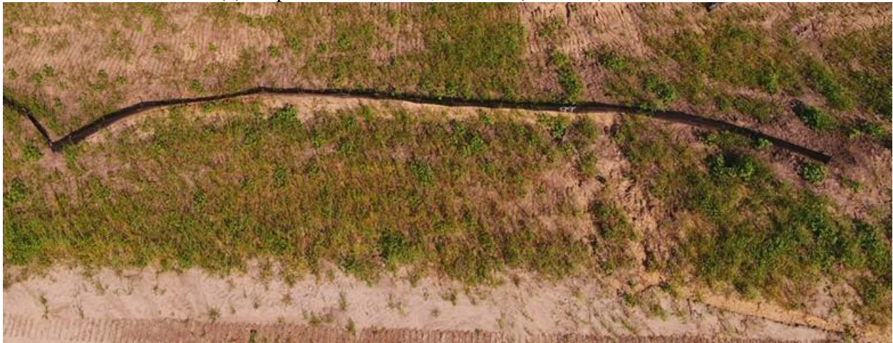
(b) Inspection 9/5/2019, 3.53 in. (8.97 cm) rainfall
