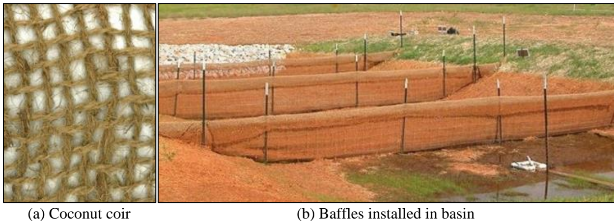
Figure 6.3. Sediment basin baffles
