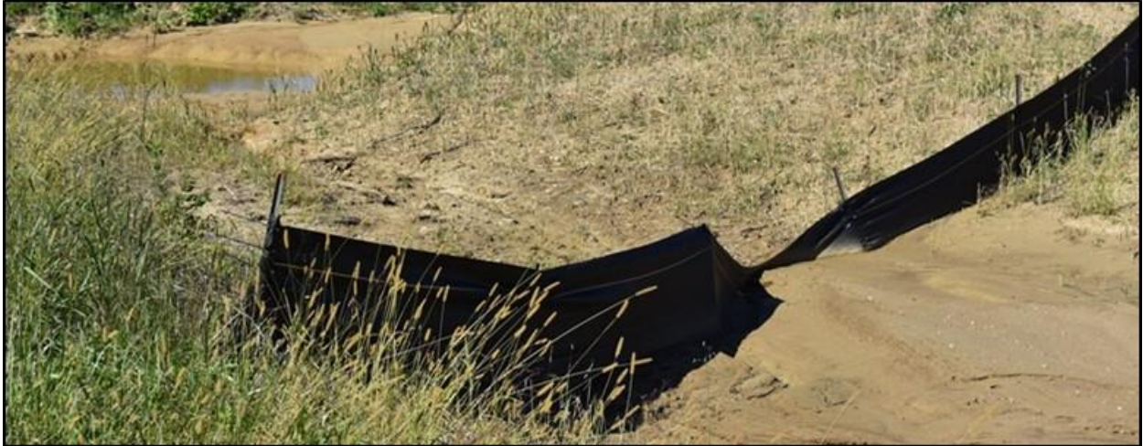
(a) Overtopping and T-post deflection
