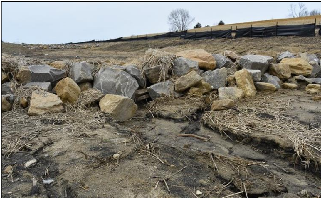
Figure 4.30. Rock check dam undercutting
