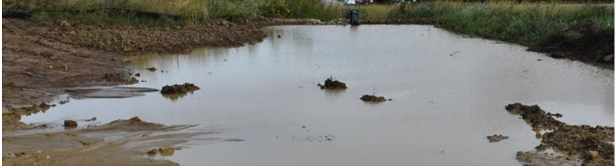
(a) Side wall sloughing and no defined inflow channel
