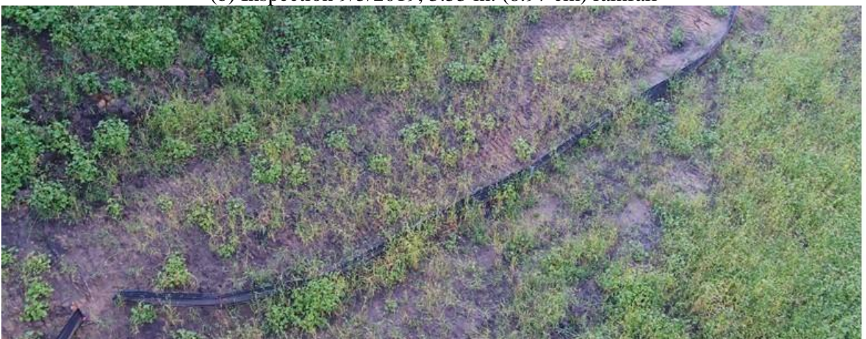
(c) Inspection 9/24/2019, 6.78 in. (17.22 cm) rainfall
