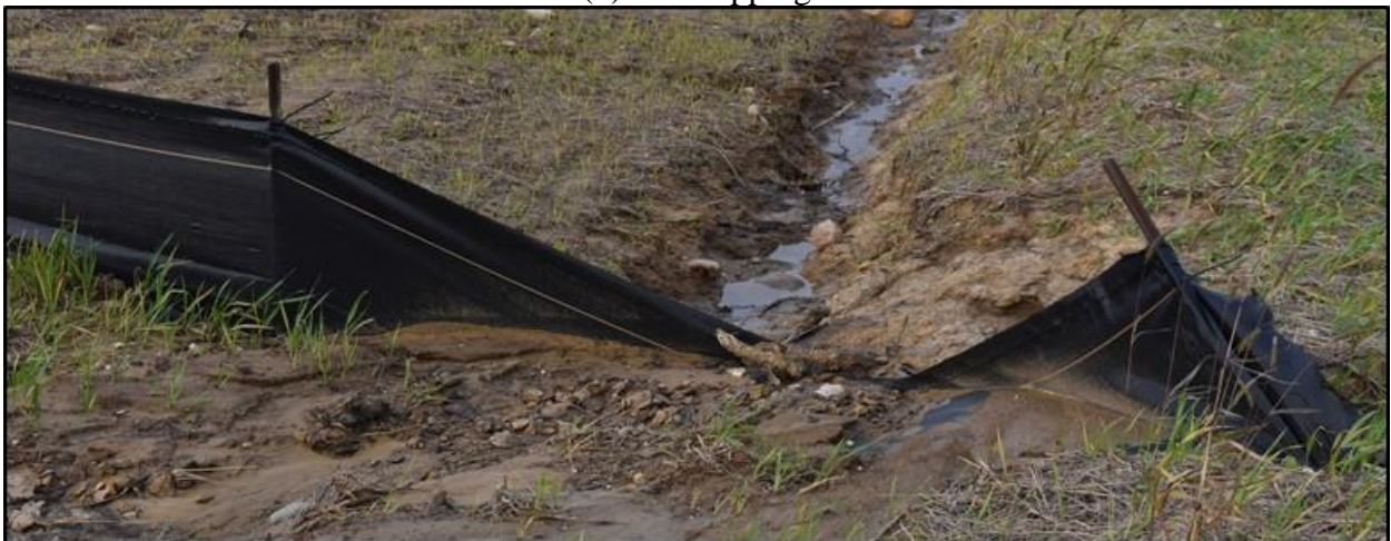
(c) Flow bypass of silt fence ditch check
