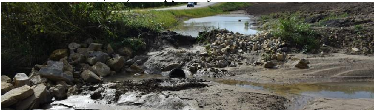
(d) Washout of berm, riser pipe discharge elevation higher than inflow, sedimentation prior to dewatering
