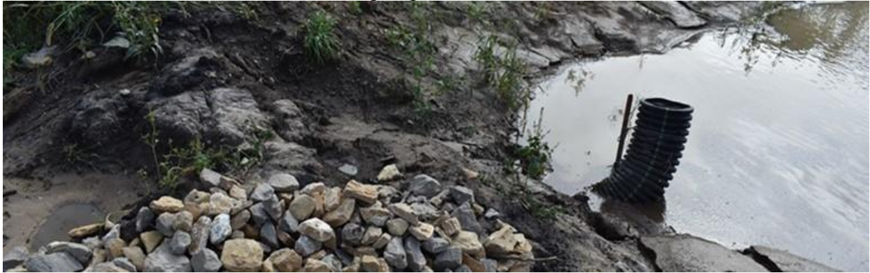
(b) Erosion of overflow berm
