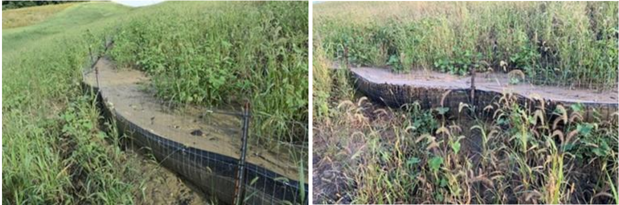
(a) Full sedimentation, no deflection (9/5/2019) (b) Overtopping due to full height sedimentation (9/24/2019)
