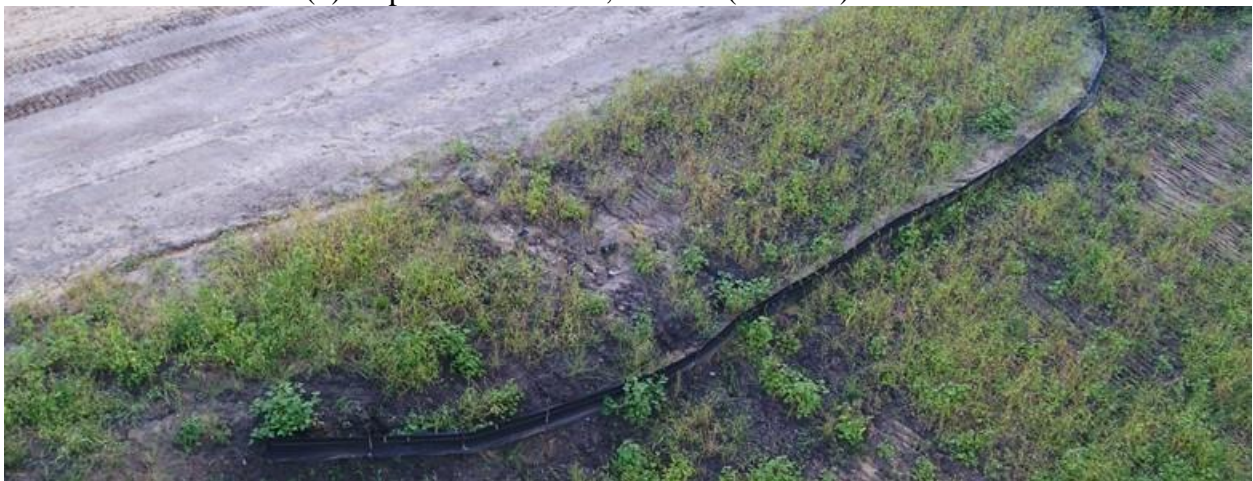
(c) Inspection 9/24/2019, 6.78 in. (17.22 cm) rainfall
