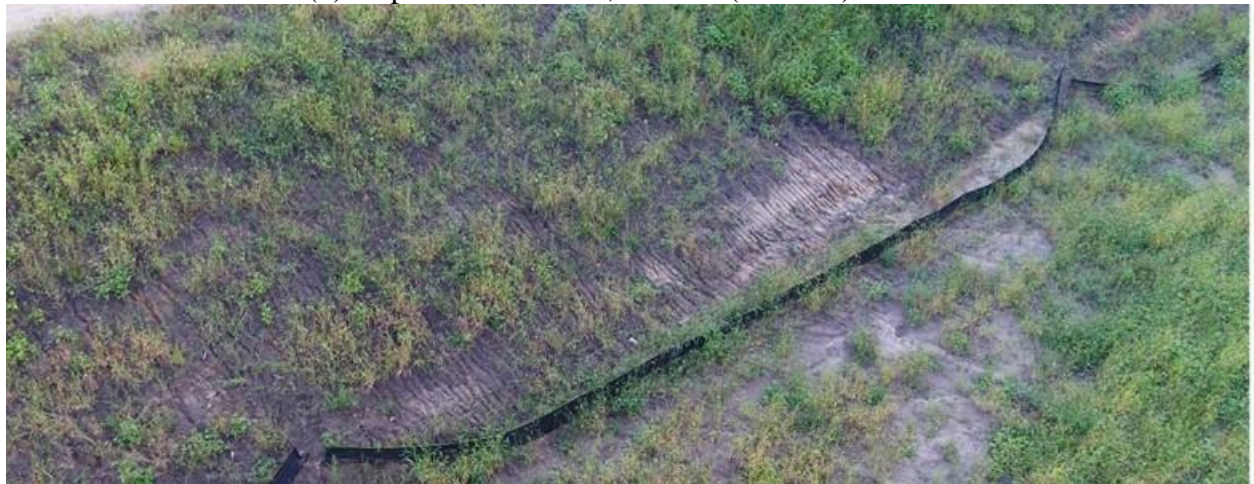
(c) Inspection 9/24/2019, 6.78 in. (17.22 cm) rainfall
