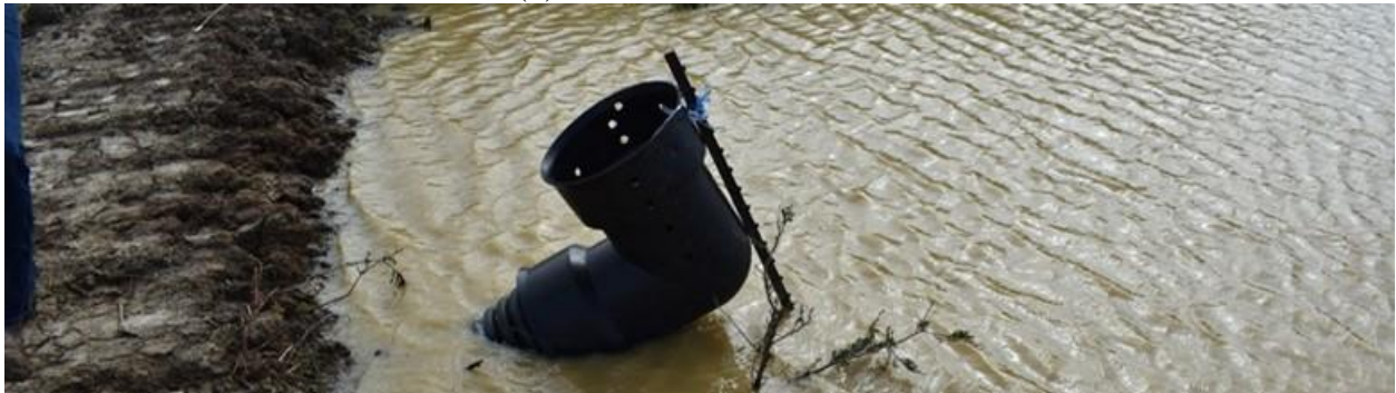
(c) Buoyant riser pipe dislodged from basin bottom
