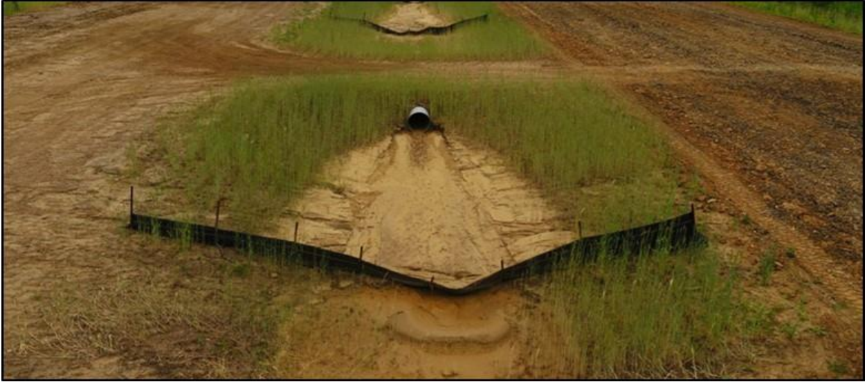
Figure 4.13. Silt fence ditch check overtopping due to T-post deflection
