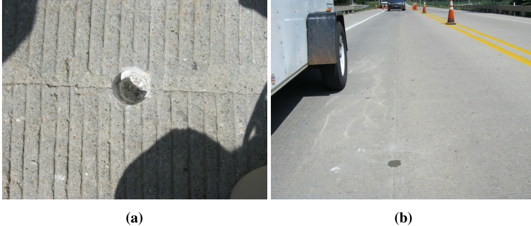
Fig. 4.2. Photographs of a hole made for chloride sampling (a) and the patched hole (b) after sampling was complete.
