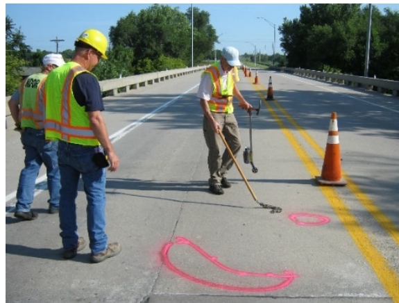
Fig. 1.1. State of the practice chain drag inspection on a bridge deck on which the locations of delaminations are marked using a handheld paint sprayer
