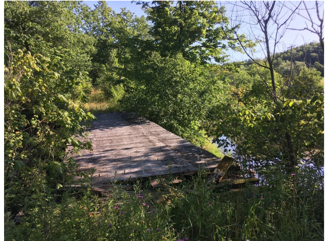
View to north (from rail trail) over bridge deck, 7/24/2019. Note collapsed decking in foreground.
