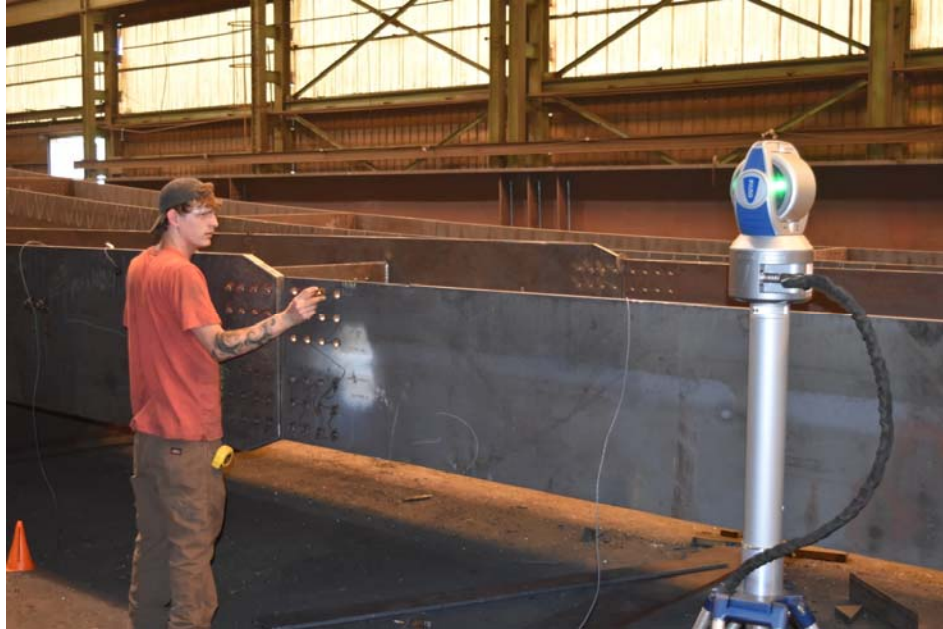
Figure 2: Measuring the locations of the splice connection holes in the girder flange with the laser tracker
