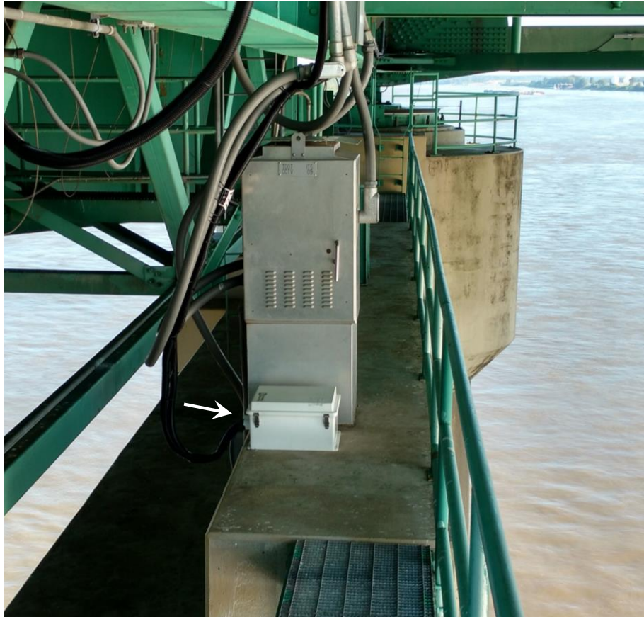
Figure 26. Data Acquisition System at Pier A (Pier C similar)
