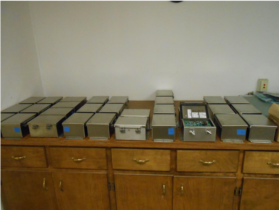
Figure 10. Episensor packages deployed on the bridge.
