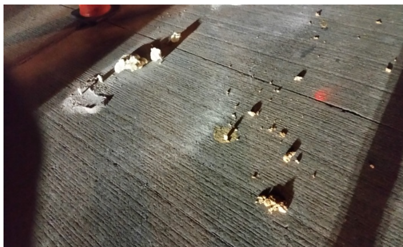
Figure 3.8 Injected PolyLevel ® material sipping out mud/water under the slab.
