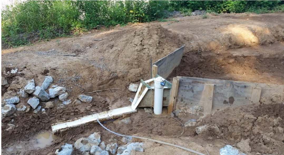
Figure 2.6. Morgan County sediment basin inlet monitoring flume and accompanying materials.
