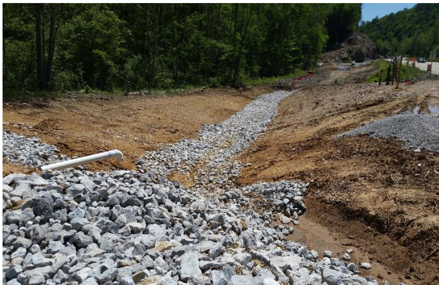
Figure 2.3. Morgan County sediment basin outlet and downstream condition.
