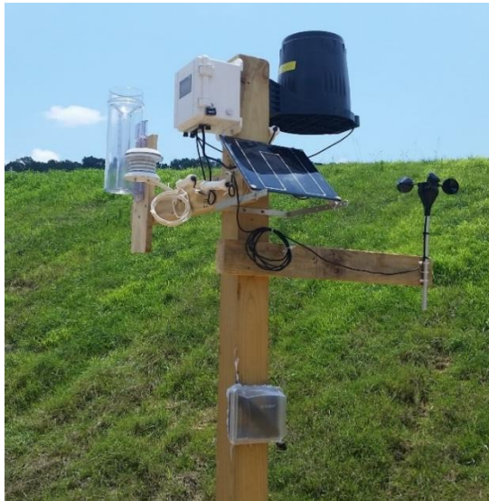
Figure 2.11. Knox County sediment basin weather monitoring set-up, includes data logger, tipping bucket rain gauge, temperature/relative humidity sensor, wind speed sensor, solar panel, manual rain gauge, and atmospheric pressure transducer.
