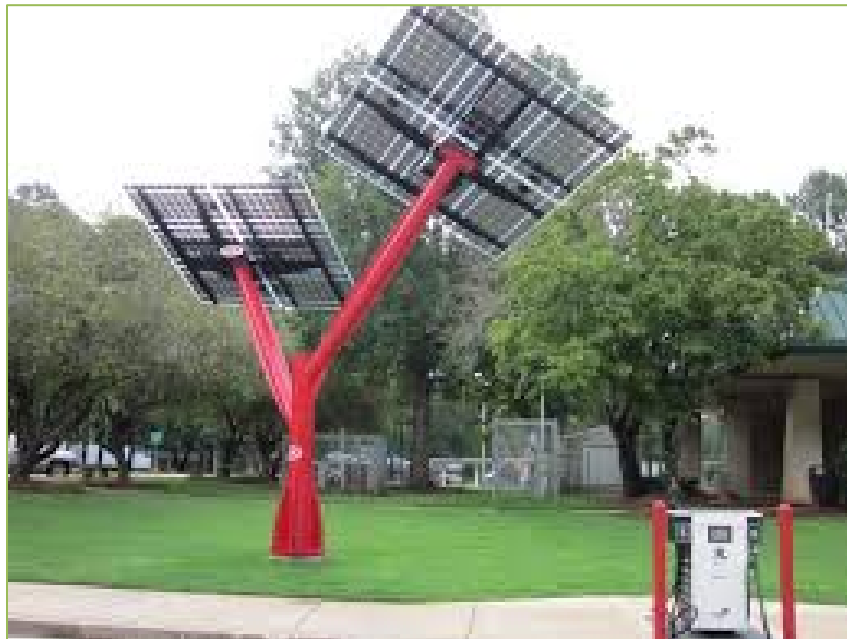
Figure 18: Solar Powered Electric Vehicle Charging Station on Ray C. Anderson Highway
