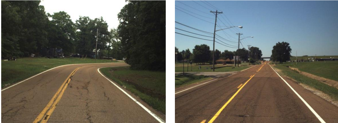
Figure 11 Typical “poor” pavement sections with low PDI
