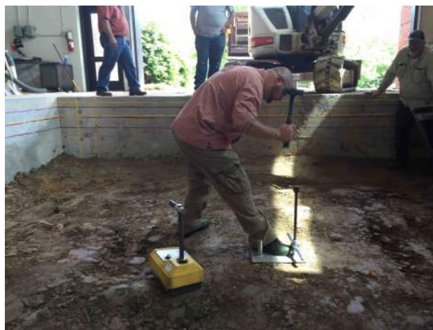
Figure 4.9: Test of Density and Compaction Degree of Subgrade Soil Using Nuclear Gauge
