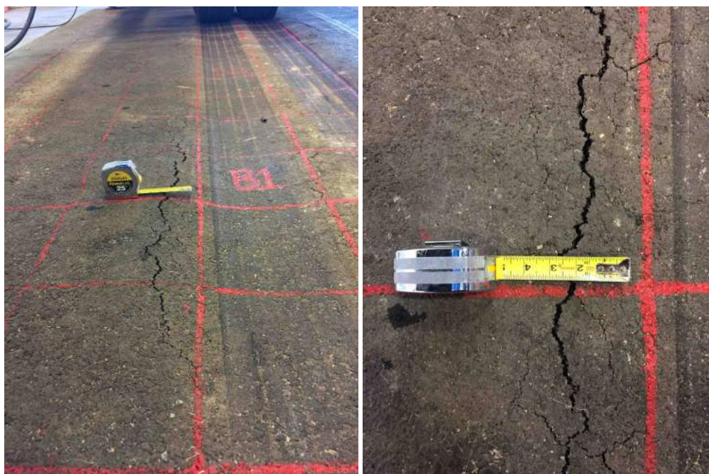
Figure 4.28: Cracks on Section with Geogrids at the Bottom of Base Layer
