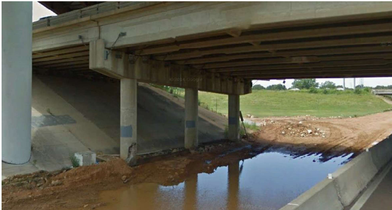
Figure 12: Example of partially open abutment vehicular access with simultaneous bridge column access to another bridge
