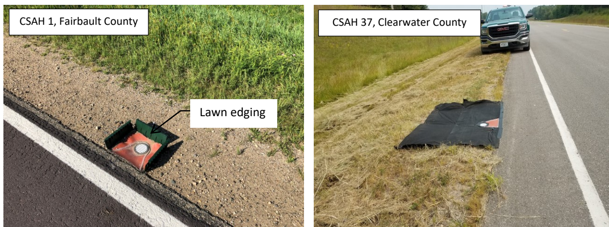
Figure 3.4 Photographs showing the installation of lawn edging (CSAH 1, Fairbault County; photo courtesy: William Goo), and geotextile fabric (CSAH 37, Clearwater County; photo courtesy: Dan Sauve) installed around the runoff sampler during 2018 monitoring. All sites were switched to geotextile fabric cover in 2019.
