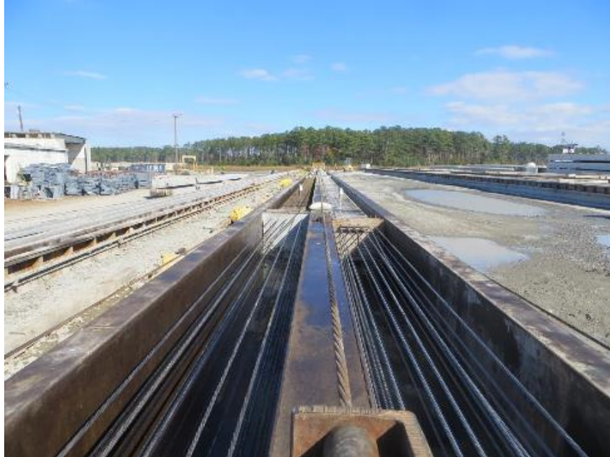
Figure 19. Preparing to Make 24-in-Square Prestressed Concrete Piles. Conventional steel strand shown on the left and 2205 stainless strand shown on the right in a 400-ft-long bed. Not shown are the steam curing pipes that lay adjacent to the bed near the ground.
