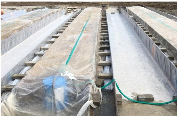
(a) Simple steel forms to cast planks (photo taken at the Midwest Underground Casting Facility in Nebraska)
