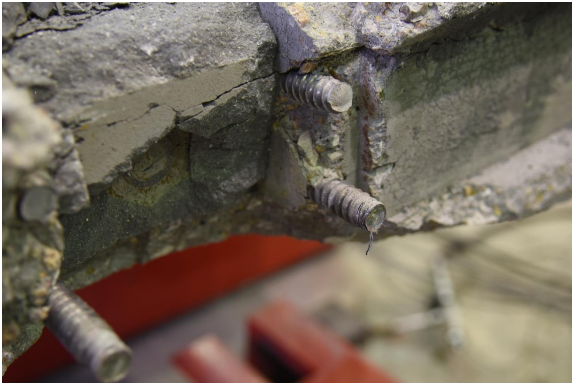
Figure 3.24: Mechanical Joint Shear Failure (Specimen C-C-1)
