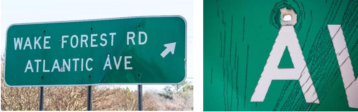
Figure 1.5 Example of damaged Signs: Scratched and Gun Shot
