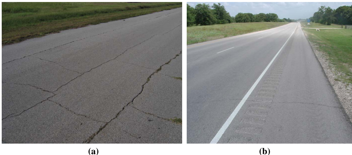
Figure 2-3: (a) Block Cracking and (b) Transverse Cracking in HMA with Stabilized Base Materials (Sebesta and Scullion 2004).
