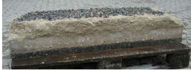
Figure 2-4: Separation between Asphalt and Cement Stabilized Base (Thogersen et al., 2004).
