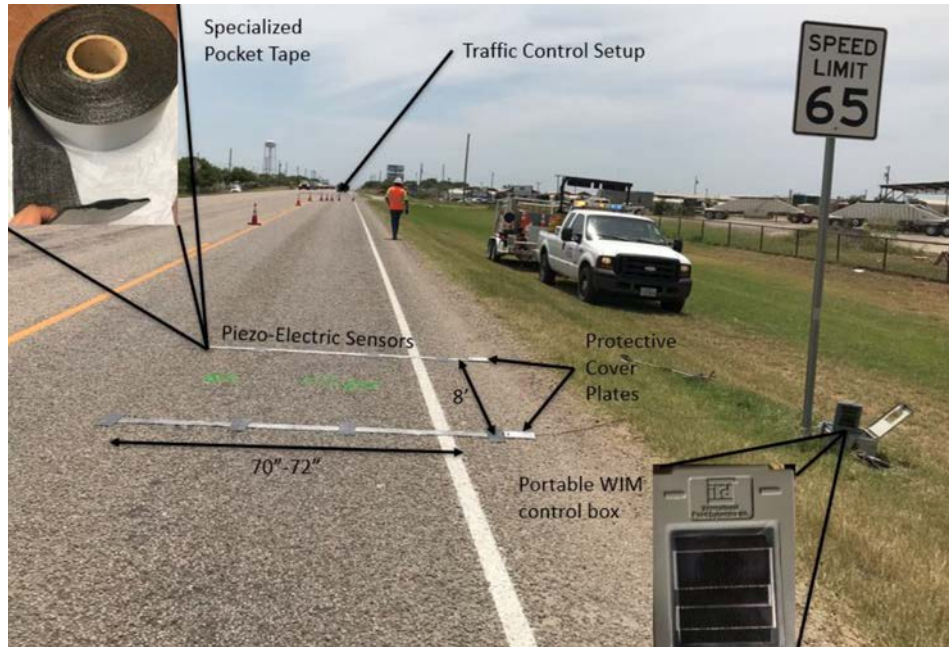
Figure 13-4: Portable WIM Equipment Setup for Traffic In-Situ Measurements.
