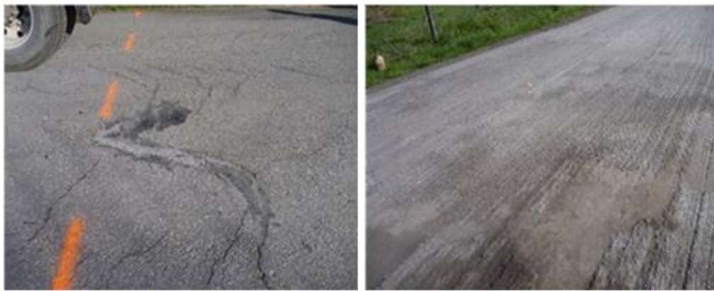
Figure 1. Slippage Cracks and Milled Surface on Route 611
