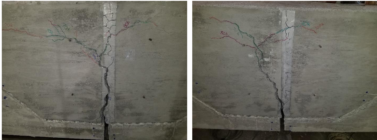
Figure 52. No Connection Specimen with Good Surface Roughening at Failure Load of 130 kips (East Side Left and West Side Right)
