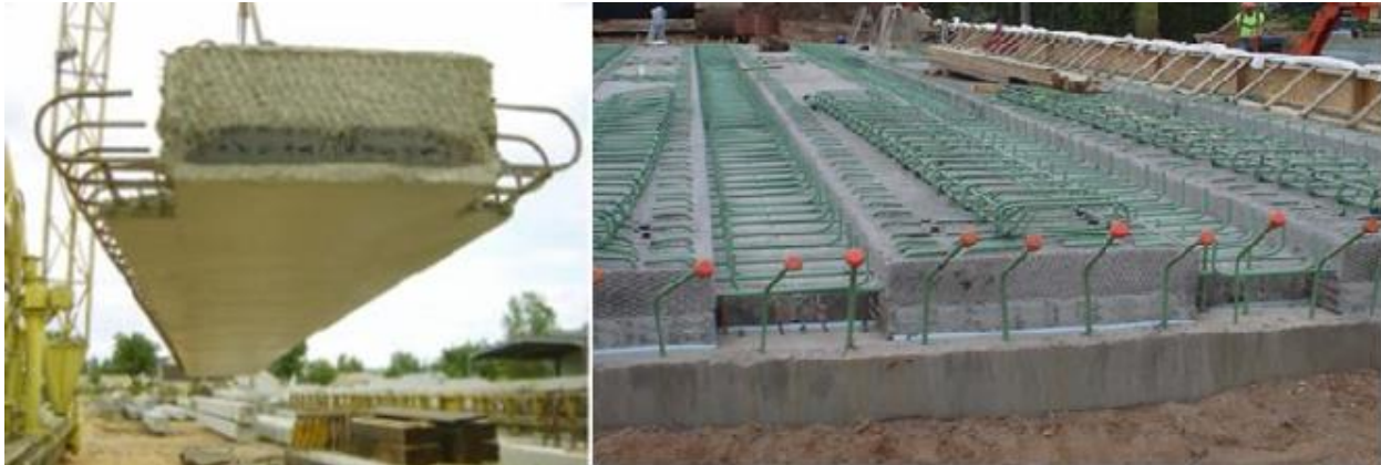
Figure 1. Development of the Inverted T-Beam System, Original Poutre-Dalle System left (reprinted with permission from Matiere, from their website at https://www.matiere-tp.com/beam-slab ), MnDOT System right (Hagen et al., 2005, reprinted with permission)
