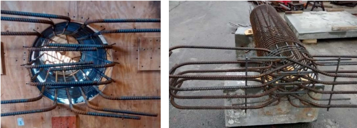
(a) (b) Figure 3-4. (a) Column longitudinal bar tails; (b) Footing “Z” bars and column cage
