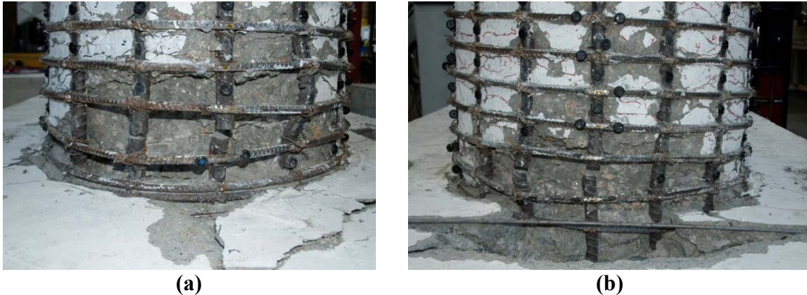
Figure 4-7. (a) South side final damage state; (b) North side final damage state
