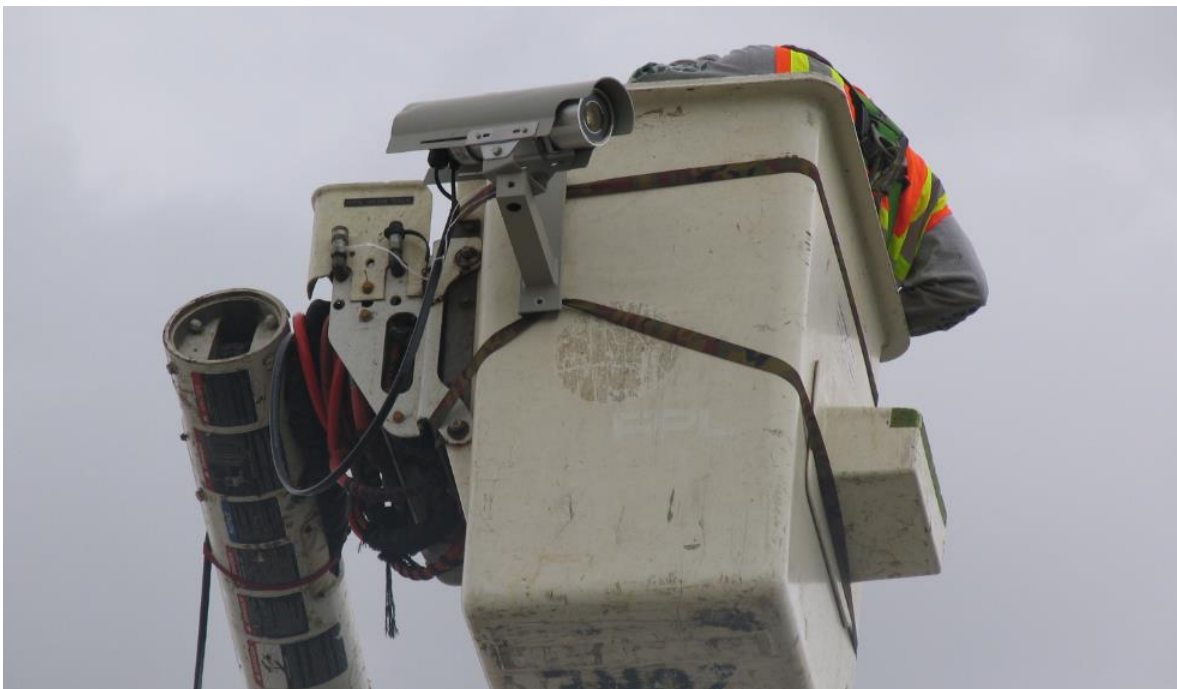
Figure 4-6. ITERIS Camera Installed on Bucket
