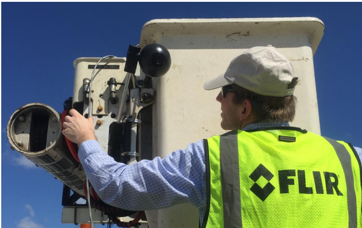
Figure 4-10. FLIR Camera Installed on Bucket
