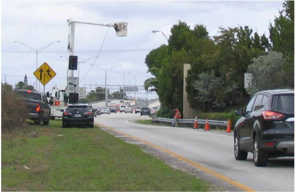
Figure 4-7. ITERIS Overhead Camera Installation over Ramp Lane
