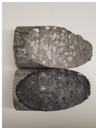
(a) Bond failure
