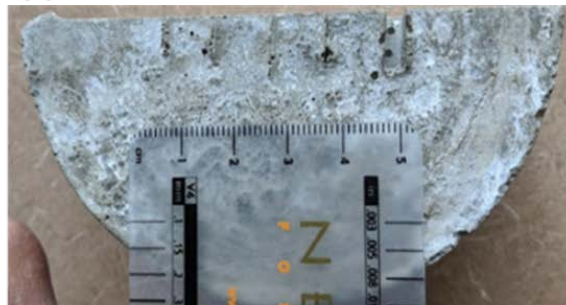
(e) Plan View of cracks
