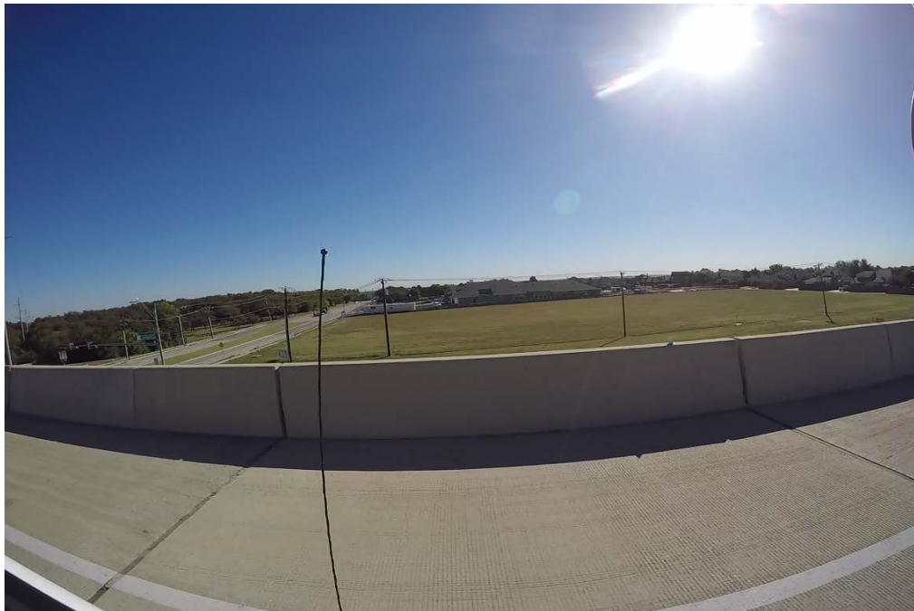
Figure 3.19: Northbound main lane. Expansion joints in the elevated section as recorded by video
