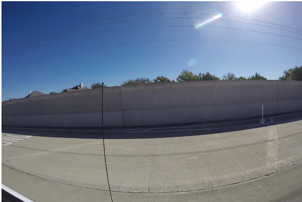
Figure 3.13: Northbound frontage road. Minor spalling of the longitudinal joint as recorded by video
