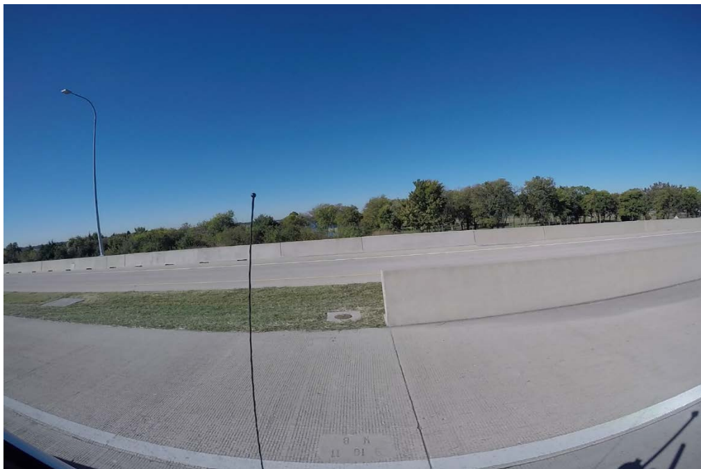
Figure 3.4: SH 190 Southbound main lane. Pavement cast on 9/10/2011 as indicated by inscription on the shoulder as recorded by video
