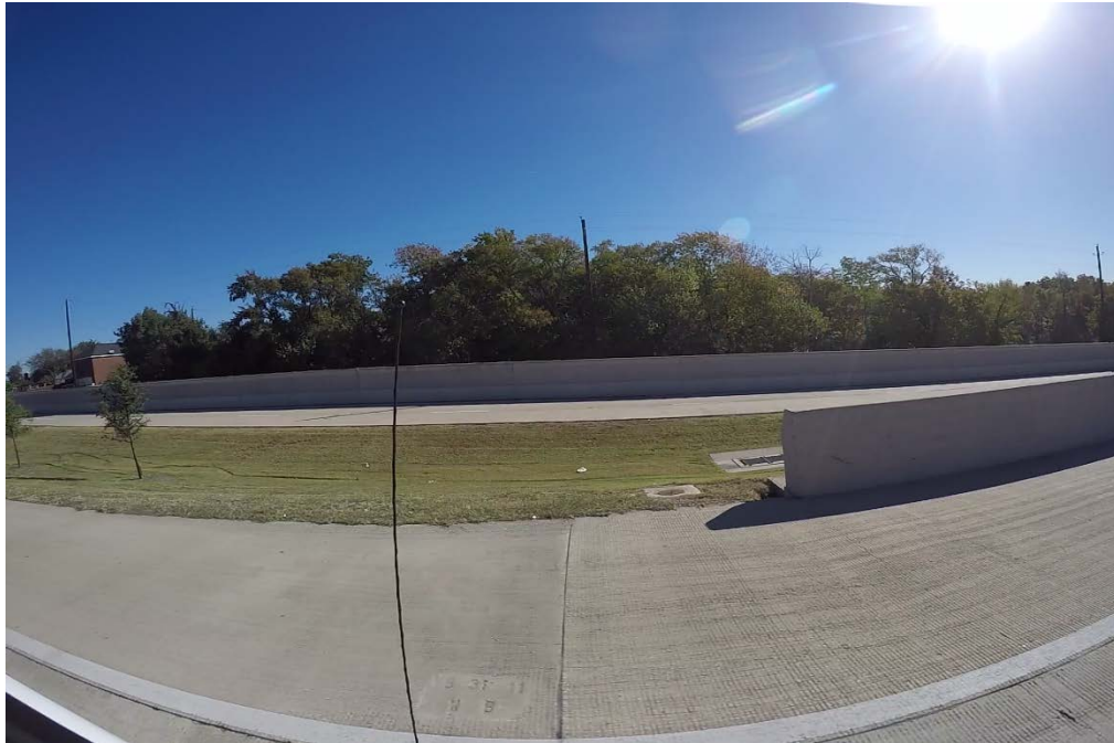
Figure 3.3: SH 190 Northbound main lane. Pavement cast on 8/31/2011 as indicated by inscription on the shoulder as recorded by video
