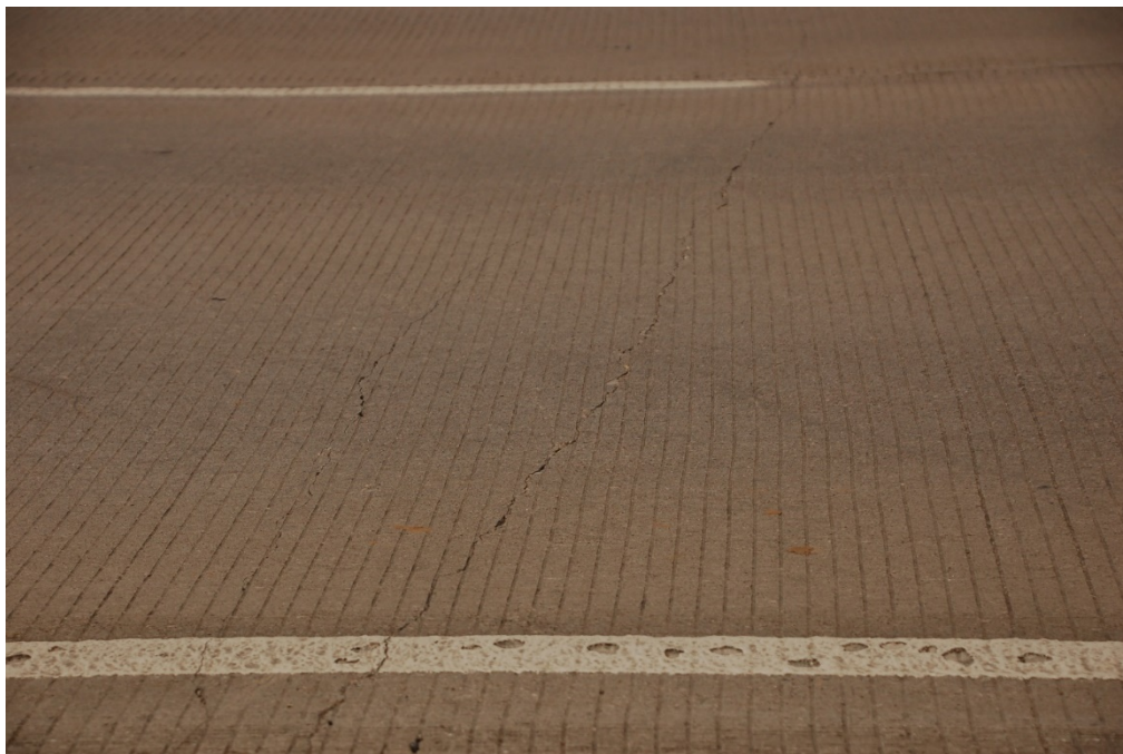
Figure 3.11: Northbound frontage road. Transverse cracks
