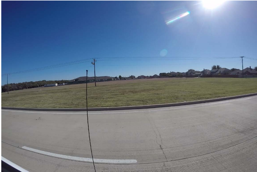
Figure 3.14: Northbound frontage road. Minor spalling of the transverse crack as recorded by video
