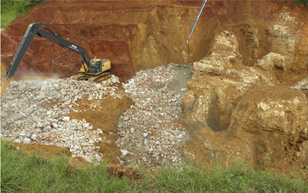
Figure 1-1: Sinkhole remediation along AL-21 in 2013 (Orange and Smith 2014).
