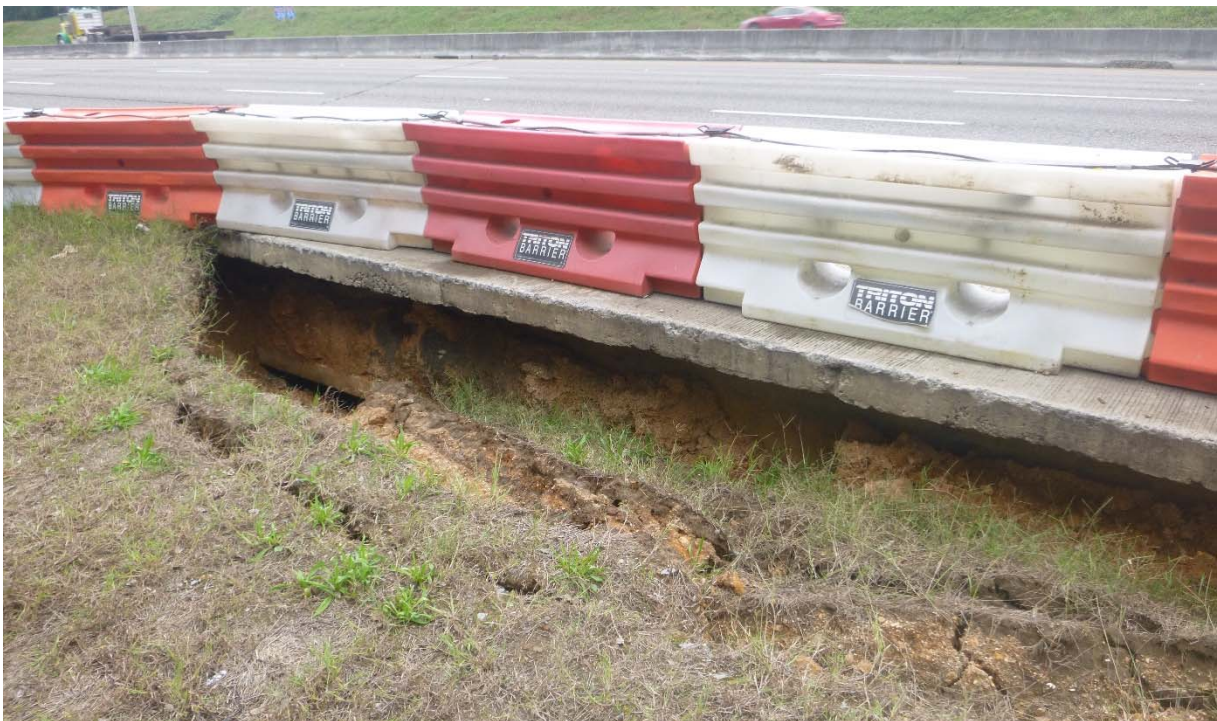
Figure 1-2: Erosion of the shoulder underneath an at-grade bridge in an area of extensive sinkhole activity along eastbound I-59/20 near Mile Marker 122.
