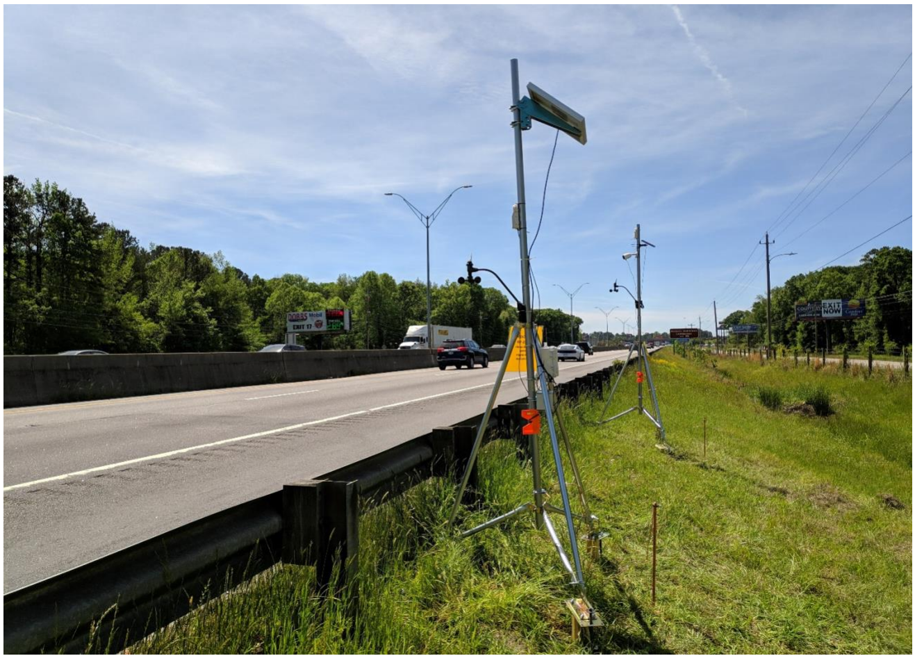
Figure 2-2 Anemometer Installation – NCDOT Highway Division 6, Interstate 95 Southbound - Lumberton, Robeson County
