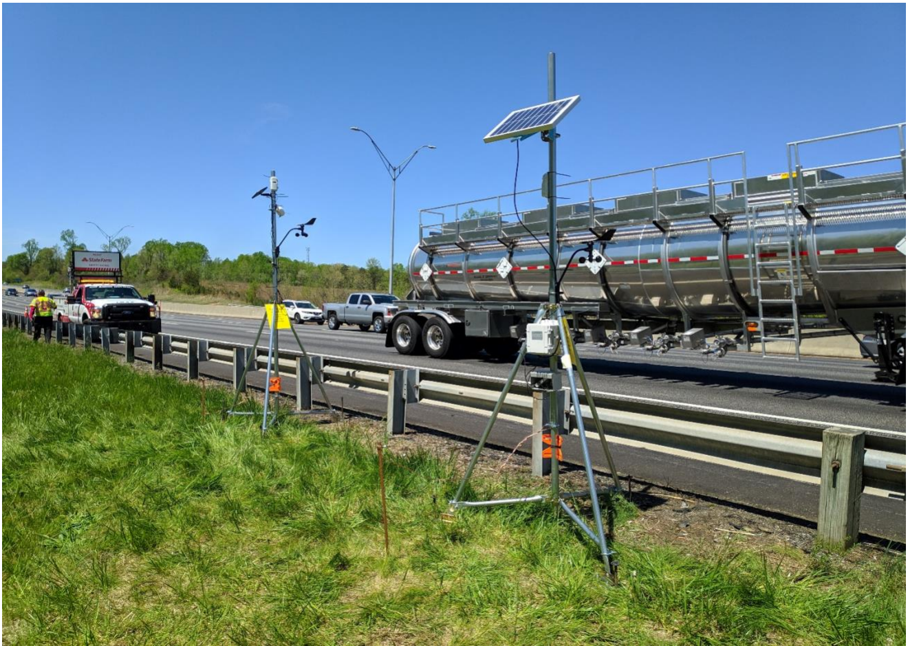
Figure 2-3 Anemometer Installation – NCDOT Highway Division 7, Interstate 40/85 Eastbound - Whitsett, Guilford County
