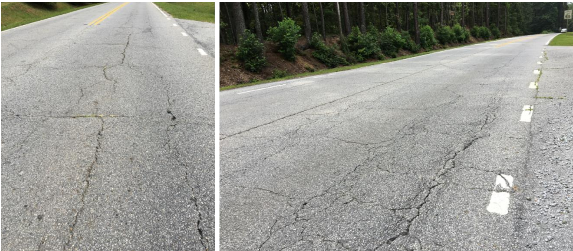
Figure 2. Photos. SR 70 pavement condition prior to rehabilitation.
