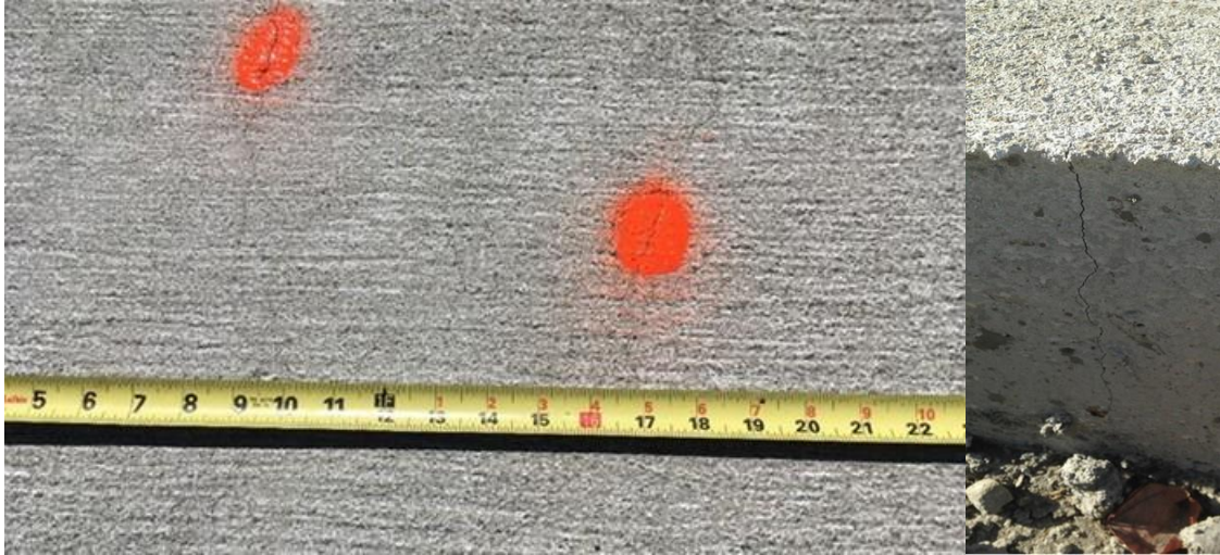
Figure 21. Crack Survey on US 60 CRCP Exposed Surface After 3 Weeks of Curing. CRCP = continuously reinforced concrete pavement.
