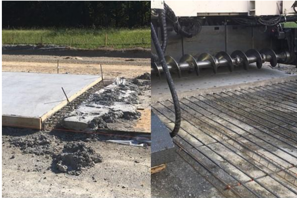
Figure 9. Construction Cold Joint With Regular Reinforcement
