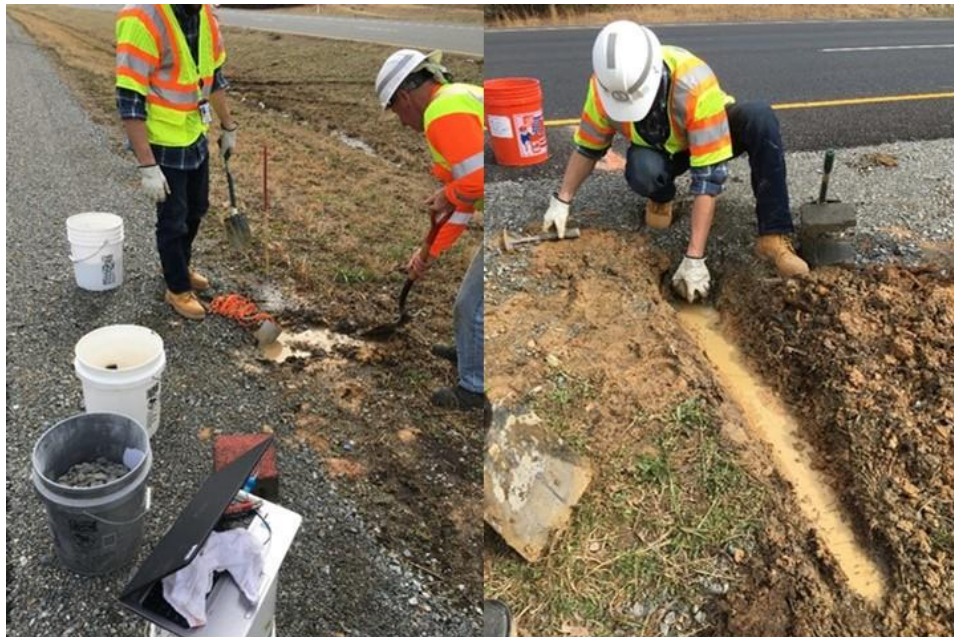
Figure 24. Standing Water at the Edge of the Pavement in February 2018
