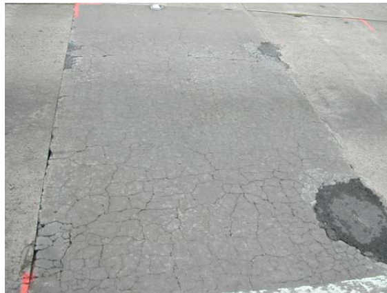
Figure 3. Cracking in full-depth repair (TxDOT, 2011)
