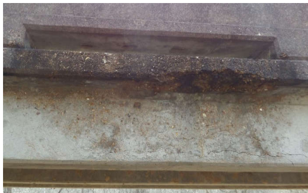
Figure 4-1. Spalling on Girder
