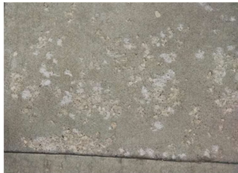
Figure 31. Salt scaling damage.
