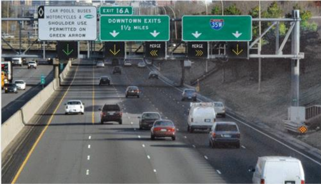
Figure 5. Intelligent lane control signals on I-35W
