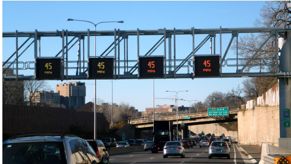
Figure 6. Active Traffic Management system on I-94 (Source: http://unge mah.com/sh_projects/i-94-managed-lanes-study-phase-1/ )
