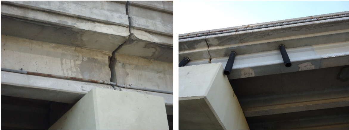
Figure 6.2: Previous Concrete Repairs to the I-244 Bridge Over the Arkansas River
