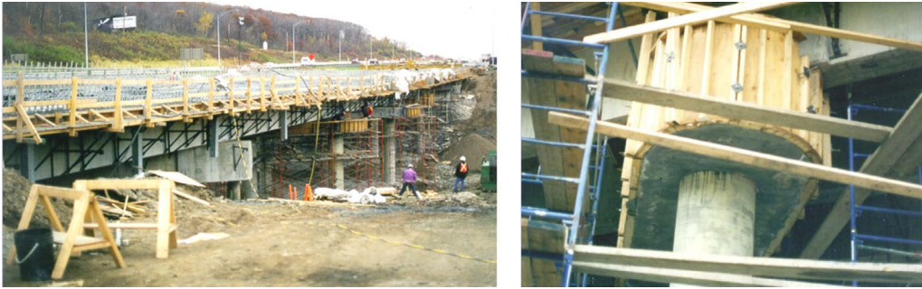
Figure 1.1: SCC Used in the Repair of Bridge Pier Caps (Khayat et al., 2010)
