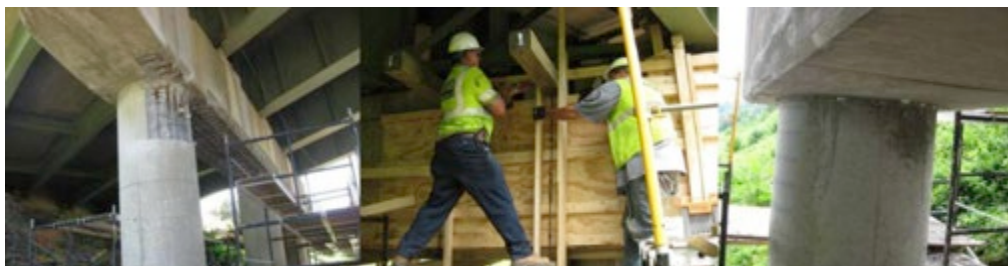
Figure 1.3: SCC Used in the Repair of Bridge Columns and Pier Caps (Ozyildirim, 2013)
