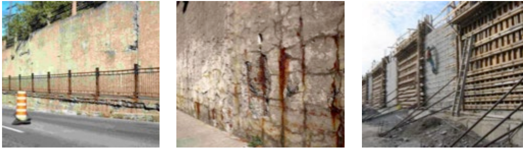
Figure 1.4: FR-SCC Used in the Repair of the Jarry/Querbes Underpass (Khayat et al., 2005)
