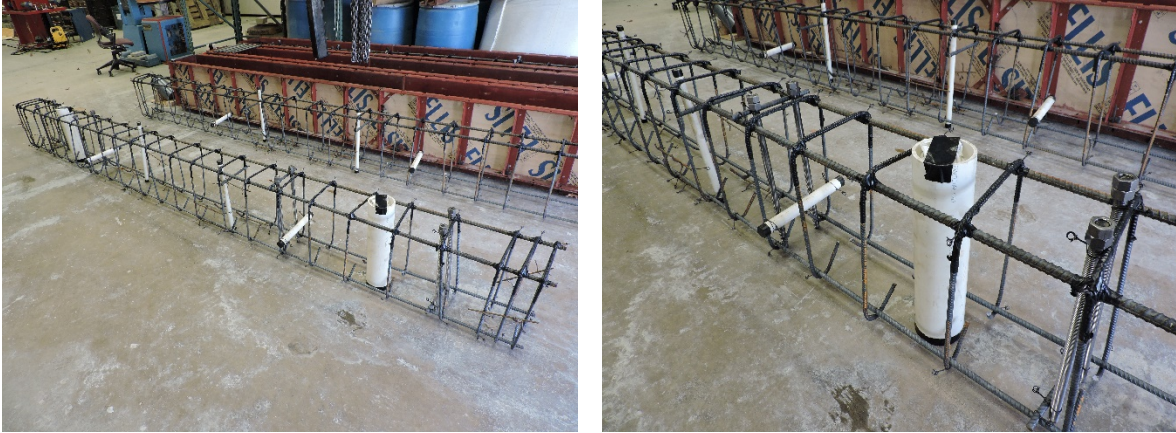
Figure 5.7: Reinforcing Cages with PVC Inserts for Access Ports, Vent Holes, and Pick Points
