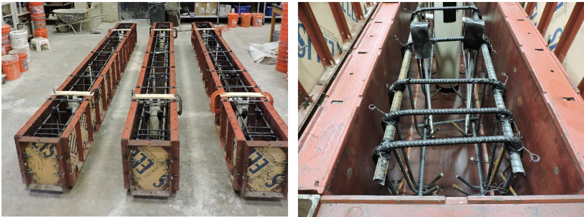
Figure 5.8: Upside Down Placement of Cages (l) and Protection of Exposed Portion of Stirrups (r)
