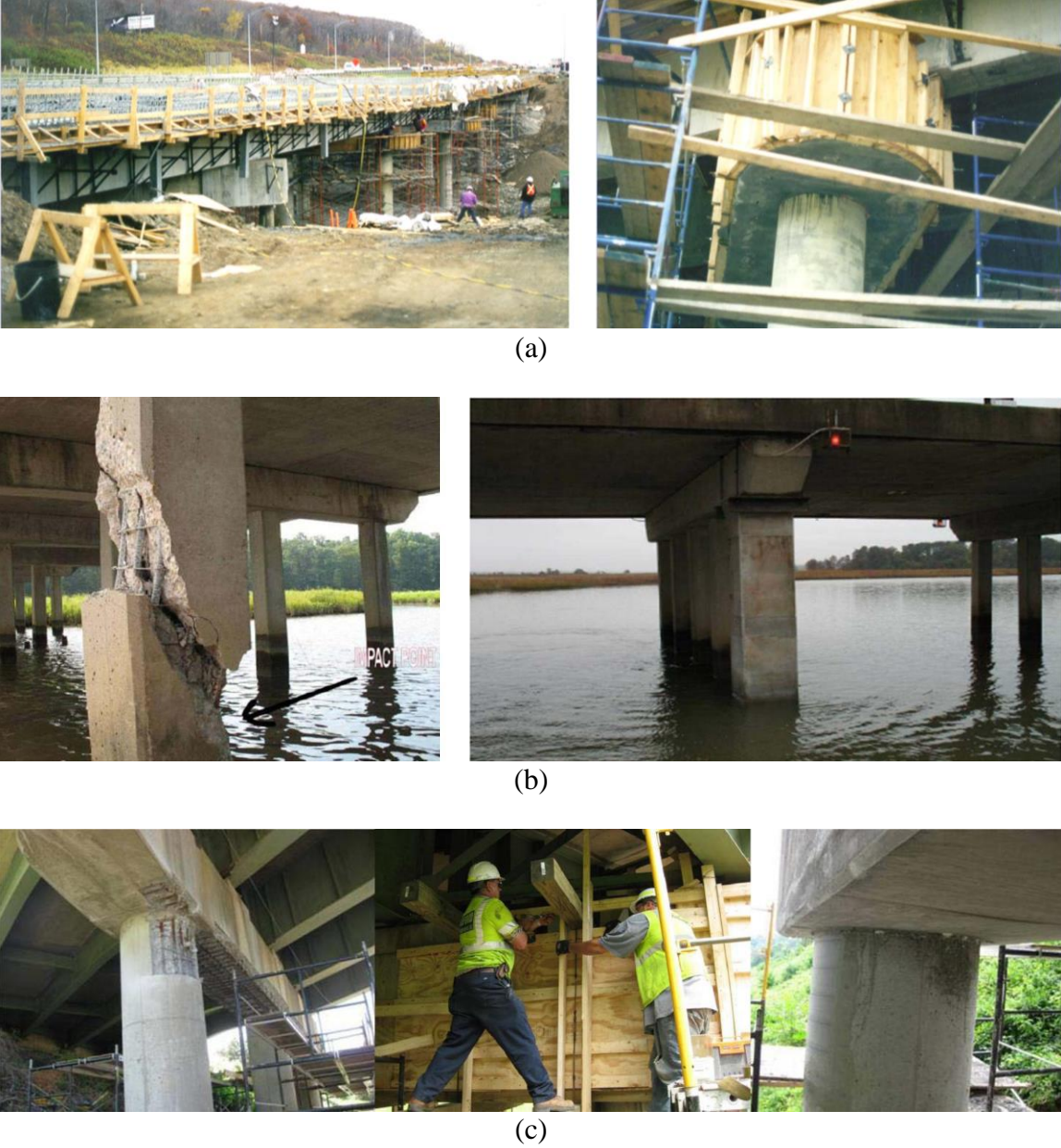
Figure 1 – Application of SCC for Repair; (a) Bridge Pier Caps and Columns in Quebec [Khayat et al, 2010], (b) Pile Damaged by a Barge in Virginia [Ozyildirim, 2013], and (c) Damaged Column and Pier Cap in Virginia [Ozyildirim, 2013].
