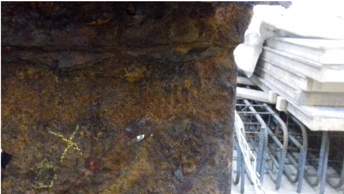
Figure 3.22: A 1/4-in. diameter hole, located 4 in. below the steel angle sections.
