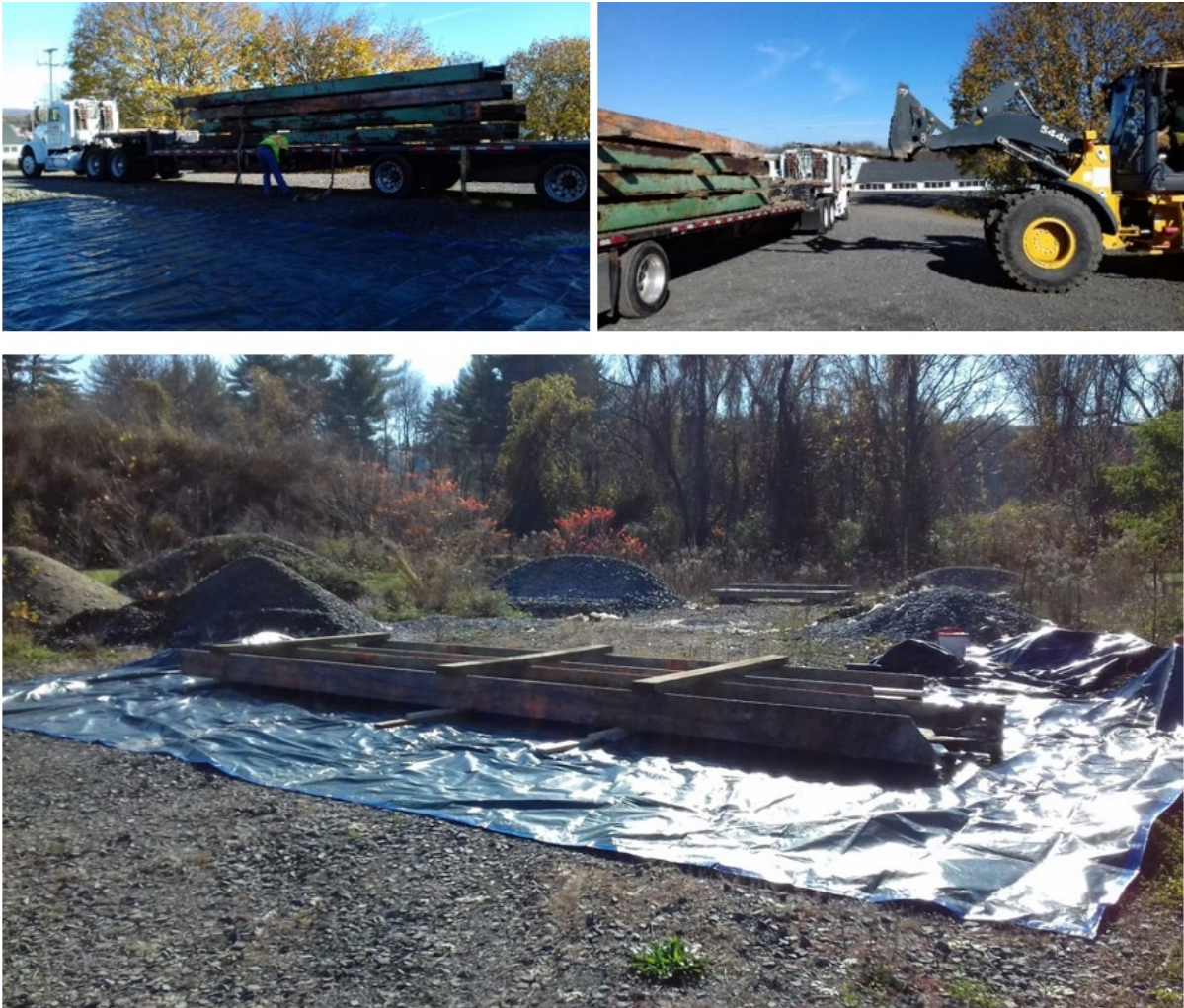
Figure 3.1: Delivery, unloading, and storage of first set of corroded beams from Colrain bridge.
