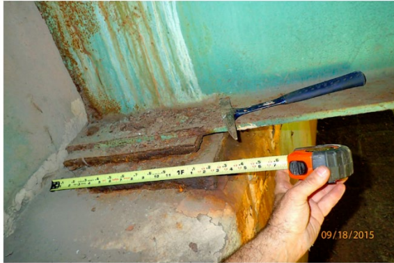
Photo 30: Typical bearing, over extended without anchor bolts.
