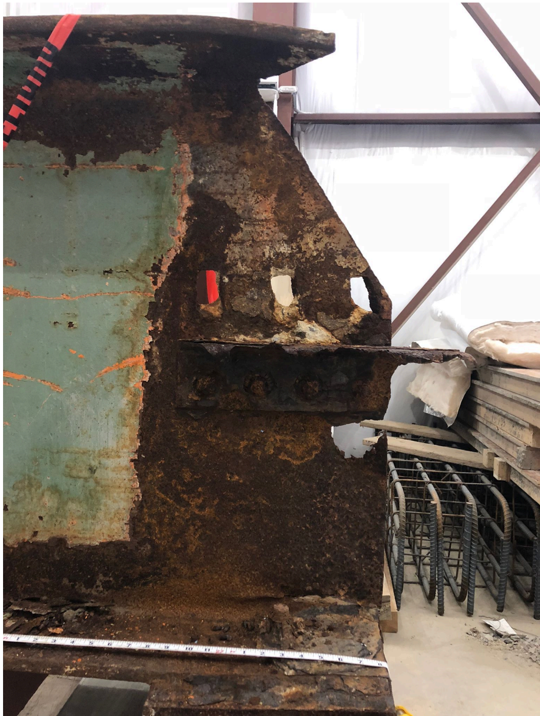
Figure 3.13: Corroded end of Specimen 1.
