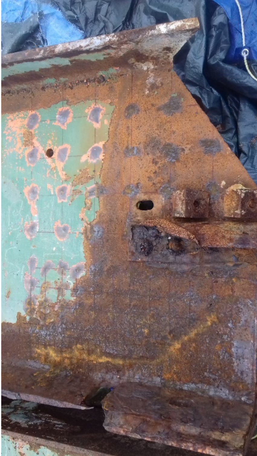
Figure 3.20: Corroded end of Specimen 2.
