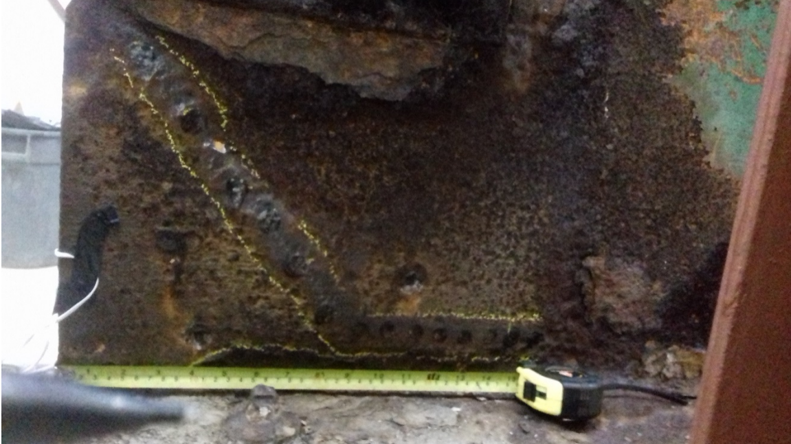
Figure 3.21: The two areas with extensive section loss at Specimen 2's web.
