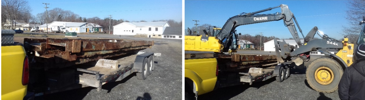
Figure 3.2: Delivery and unloading of corroded beams from Charlemont bridge.
