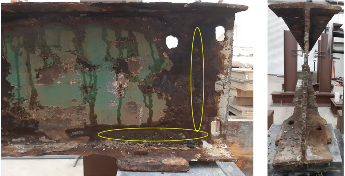
Figure 3.34: Side and front view of Specimen 4; yellow circles illustrate two areas with extensive section loss.
