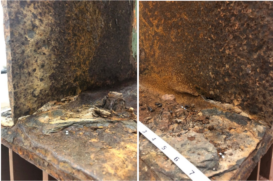
Figure 3.14: Area with 100% section loss above the flange, shown from both web sides.
