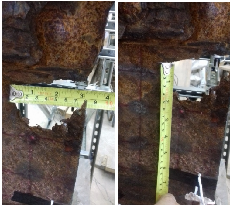
Figure 3.15: Area with 100% section loss below area where diaphragm was originally located.
