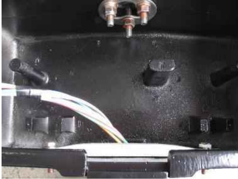
Figure 98: Disconnect box for 3-section signal with no observed damage
