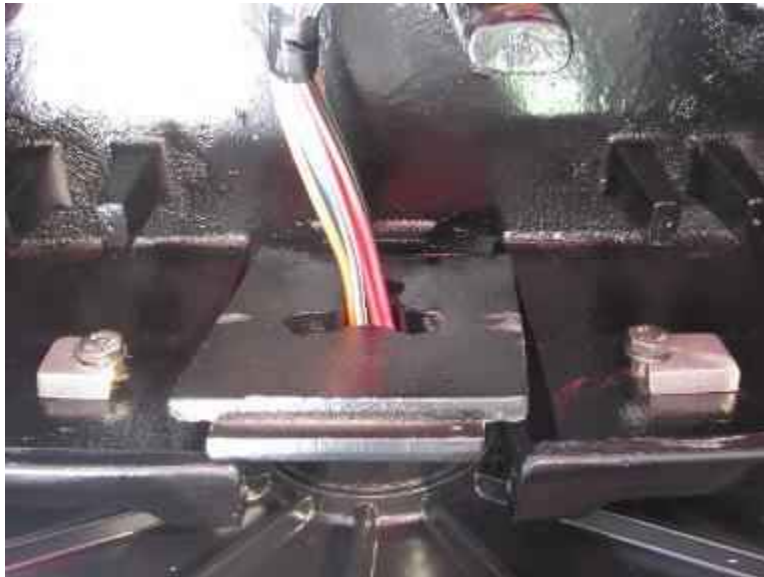
Figure 97: Cracked lower clamp inside 5-section disconnect box
