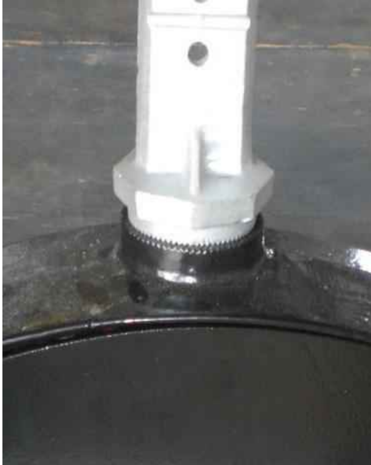
Figure 30: Serrated teeth connection between the bracket and the top of the disconnect box with no noticeable damage
