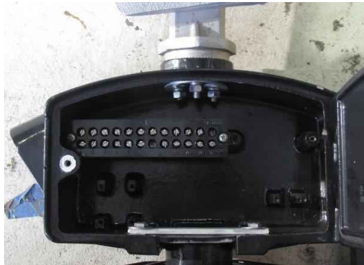
Figure 197: Disconnect box after full test (wiring was removed)
