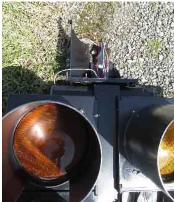
Figure 161: 5-section polycarbonate signal cracked at the top
