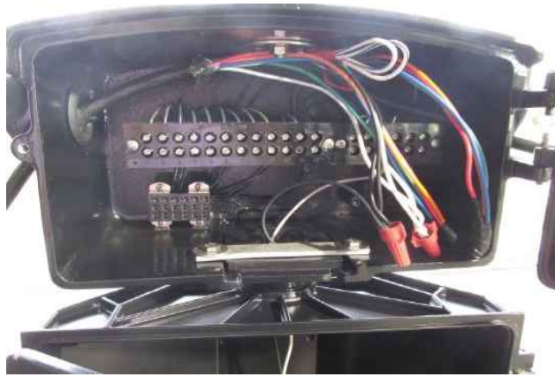
Figure 114: Disconnect box for 3-section traffic signal after test
