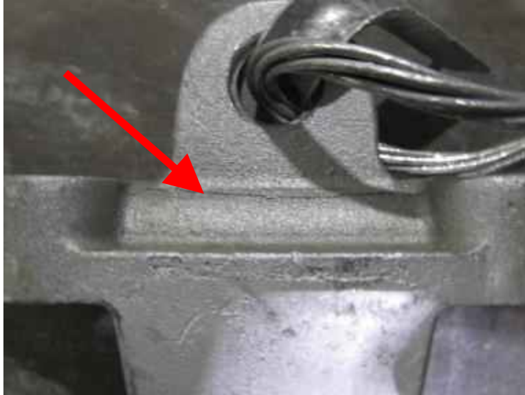
Figure 160: Hairline crack on 5-section signal messenger clamp
