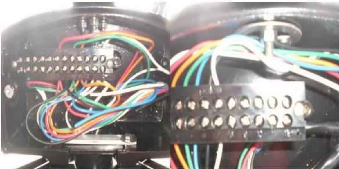
Figure 51: Disconnect box for 4-section signal after Test 2 showing no noticeable damage
