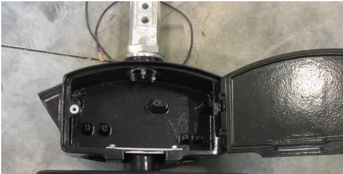
Figure 131: Disconnect box for 3-section signal with no visible damage (all wiring removed)
