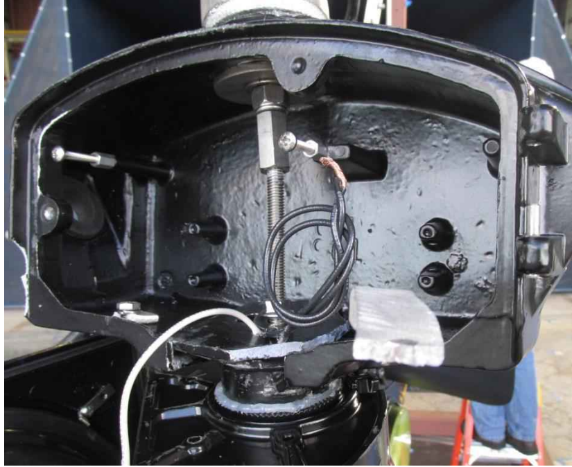
Figure 83: Disconnect box for 5-section signal after the completion of test
