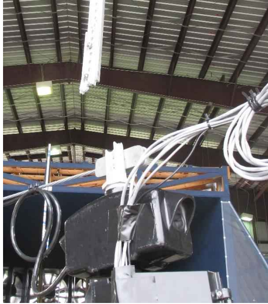
Figure 194: Fractured bracket connected to the top of the 5-section signal disconnect box
