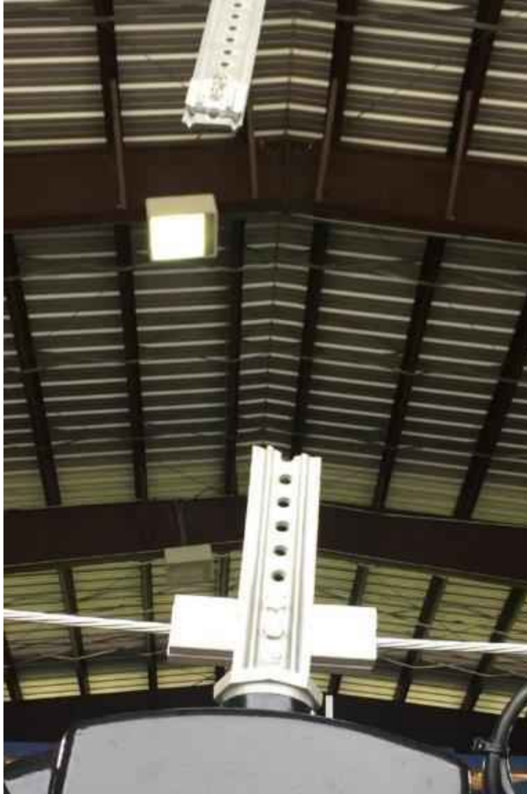
Figure 33: Tri-stud adjustable hanger after Test 1 showing location of damage. No noticeable damage to the extruded aluminum messenger wire clamp
