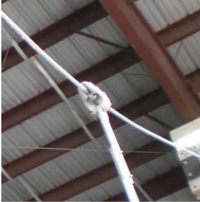
Figure 34: Span wire clamp attached to the catenary cable with no noticeable damage
